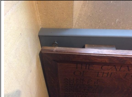
Detail view of screw fixing at upper hanging plate and with metal tube spacer to secure memorial board to secondary board support.
