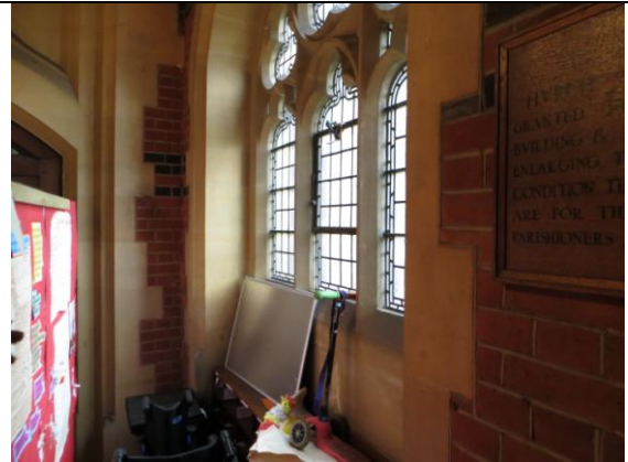
14. Overall view of likely previous location of memorial board (West window of North porch), with position towards bottom of window.
