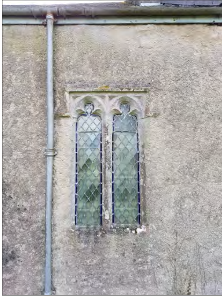
Pl. 22 General view of 14th century window with squared head and hood mould, St Mary, Rattery.
