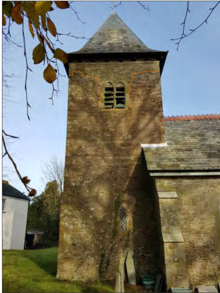
Pl. 12 General view of church tower showing 19th century rebuild (top). Looking north.
