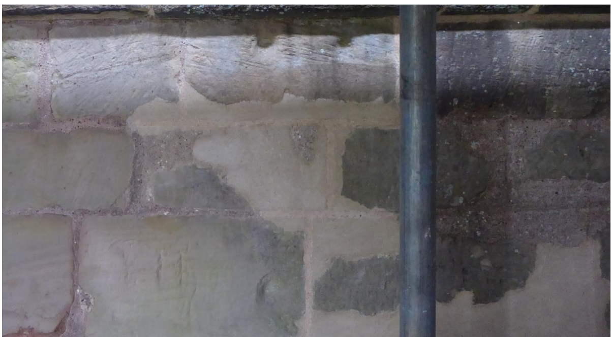
Figure 72 Condition of new mortar repairs to exterior wall
