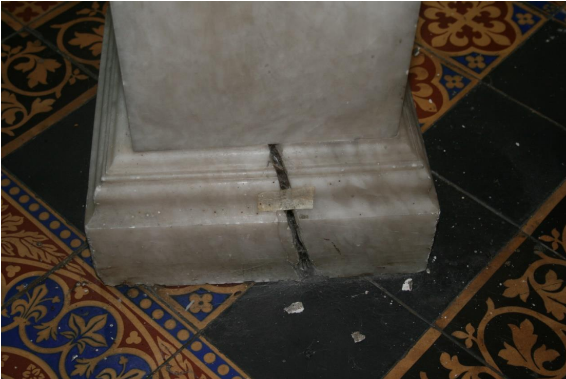
Figure 65 Initial condition of crack to the base of candlestick
