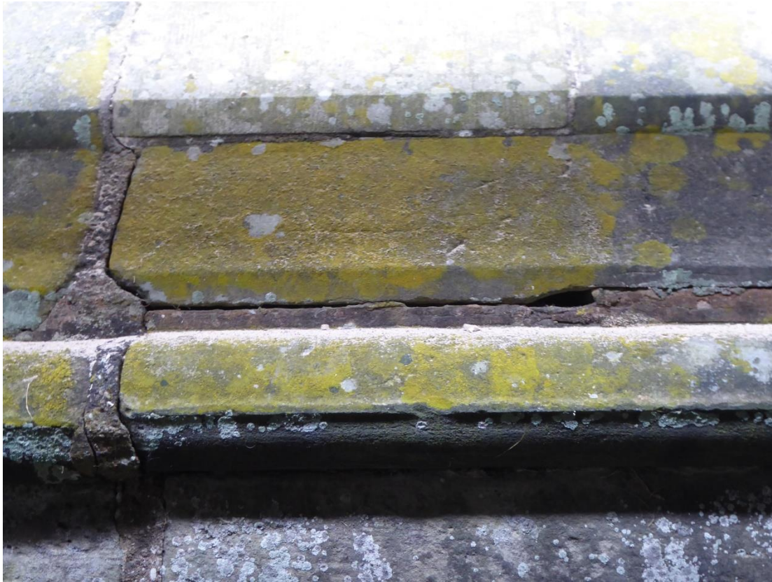
Figure 73 Initial condition of pointing mortars to exterior wall
