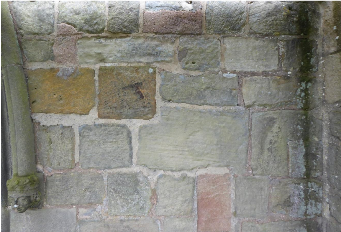
Figure 75 Initial condition of pointing mortars to exterior wall
