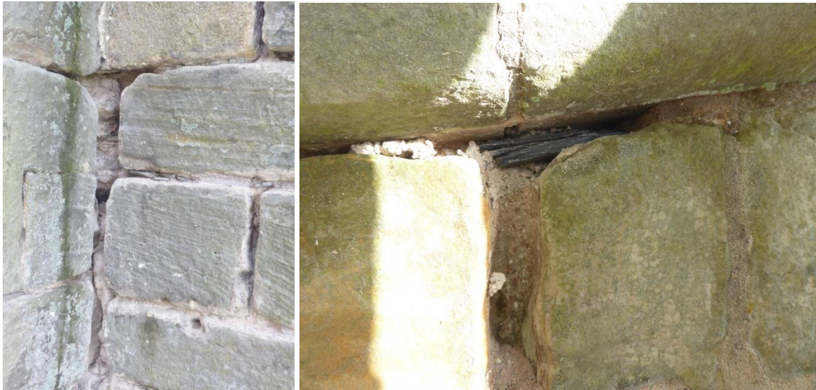
Figure 35 Failed pointing mortar raked out and filling of joints with slate fragments
