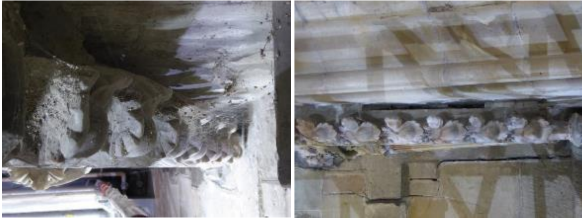
Figure 3 Dust, cobwebs and debris before and after initial dry cleaning.
