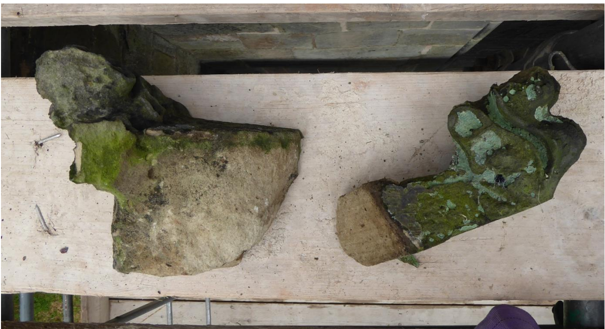
Figure 80 Fragmented pieces to south pinnacle
