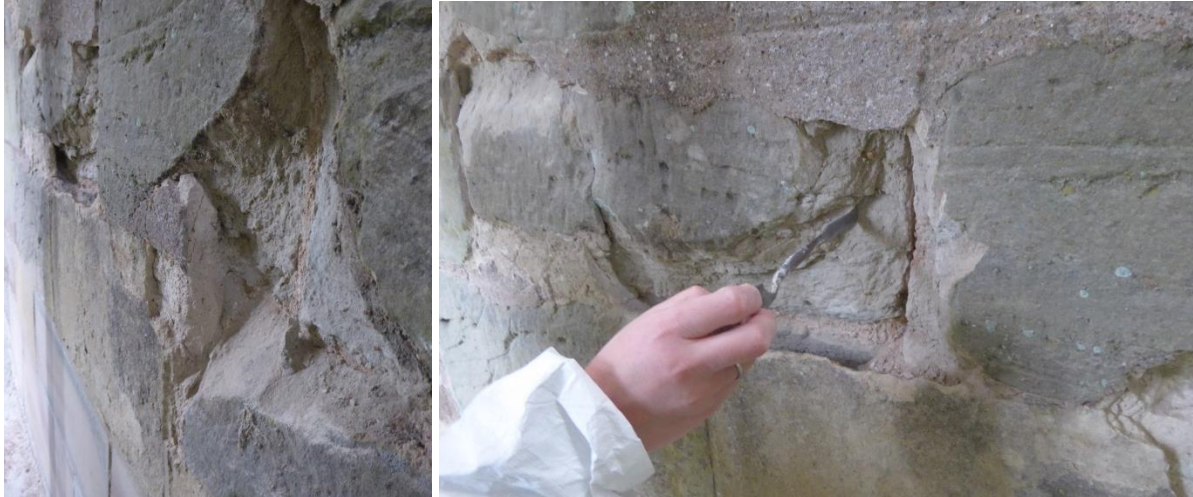
Figure 39 Removal and depth of failed previous mortar repairs
