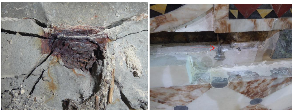
Figure 10 Condition of the ferrous cramps and cement based mortar. Replacement for stainless steel cramps
