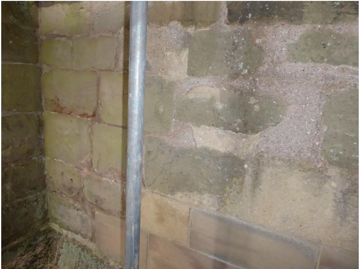
Figure 71 Initial condition of previous mortar repairs to exterior wall
