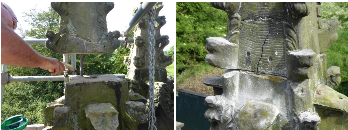
Figure 45 Relocation of the south pinnacle upper section and pinning to the north pinnacle
