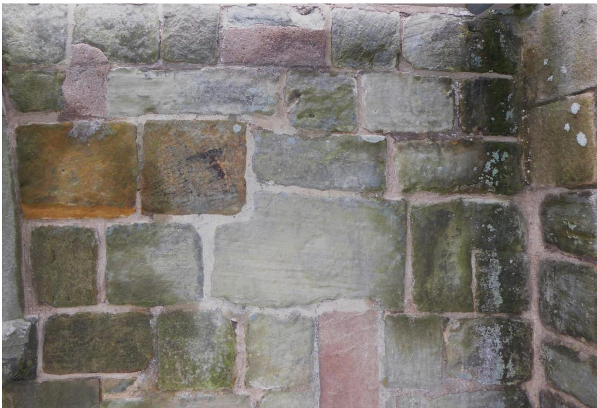
Figure 36 Wall section after the application of the base coat mortar to most of the joints
