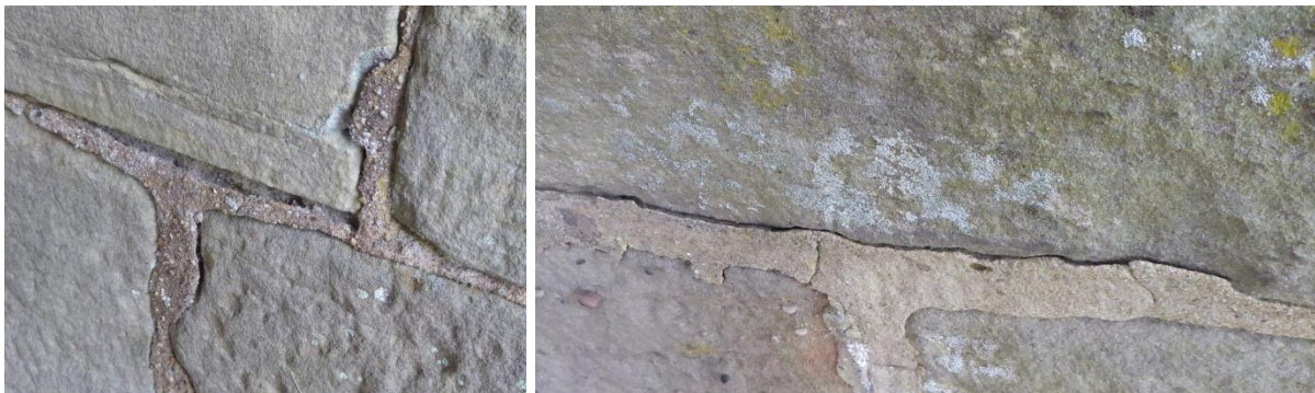
Figure 34 Examples of failed pointing mortar to the exterior wall
