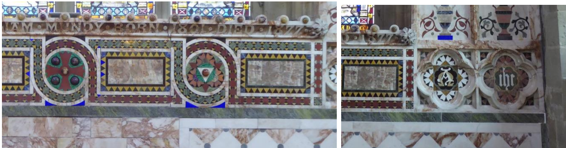
Figure 14 Location of the loose sections (blue)
