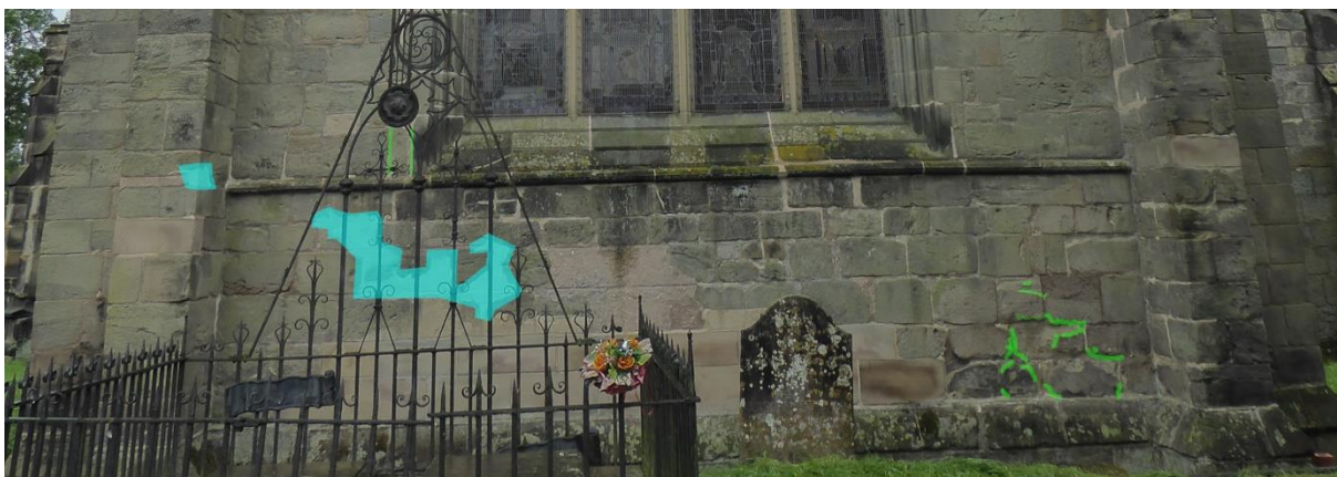
Figure 43 Location of the mortar (blue) and capping (green) repairs to the Chancel exterior east wall
