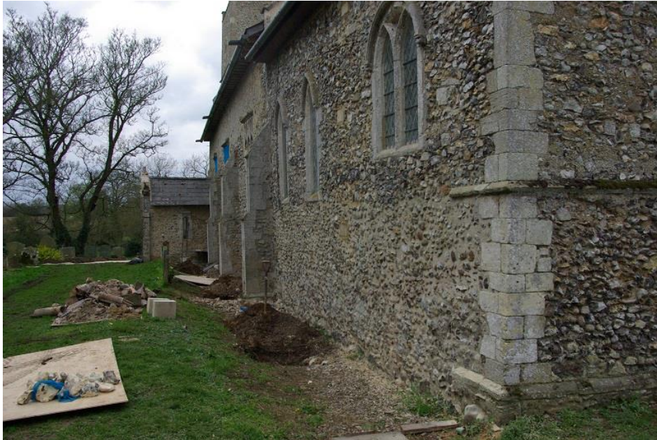
Plate 1: 'Dry area' and work in progress at S side of church, looking W
