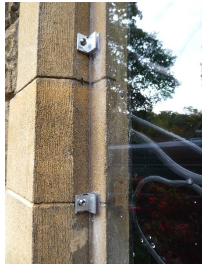
Polycarbonate protection screen held by special clips that screw into the main body of the stonework.
