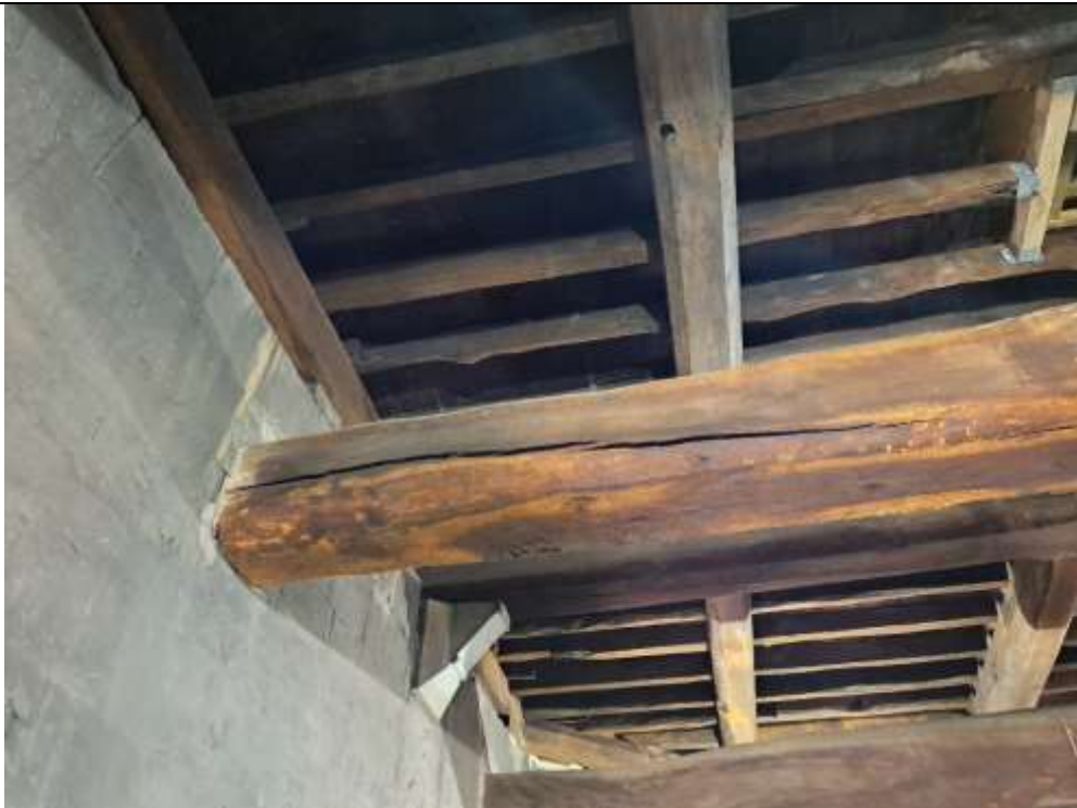
Split/crevice in ceiling beam in belfry
