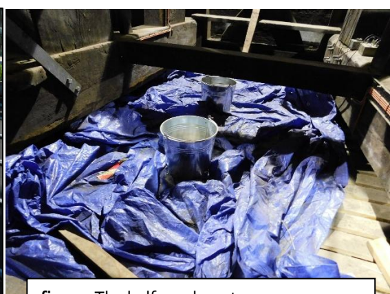
fig.03: The belfry, where temporary protections are in place to contain water ingress
