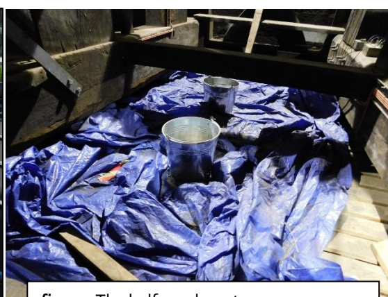
fig.03: The belfry, where temporary protections are in place to contain water ingress
