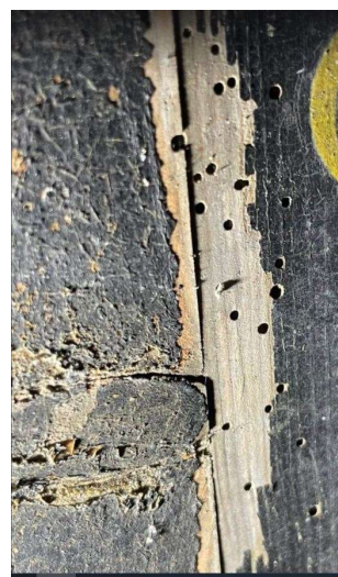
Figure 34 Shrinkage of the wood is causing gaps to the board from top to bottom. There is also a shrinkage of mainly the black paint layer area.
