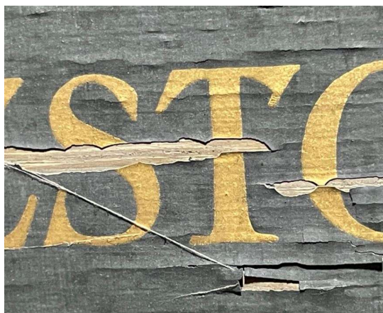
Figure 18 The commemoration black board is closer to the wall and it may be the reason for the paint lifting
