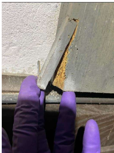
Figure 29 There are woodworm signs all over the surface of the boards but for some reason the bottom sides of the frame are the most damaged.
