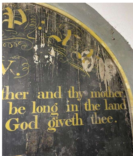
Figure 32 Loss of mainly the black surface paint on the top part of the board.
