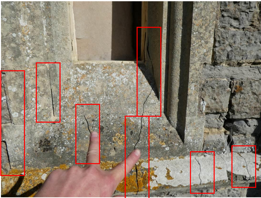
Figure 35 - P1000368 Masonry Fractures & Open Joints in 3rd Stage Window Sill South Elevation
