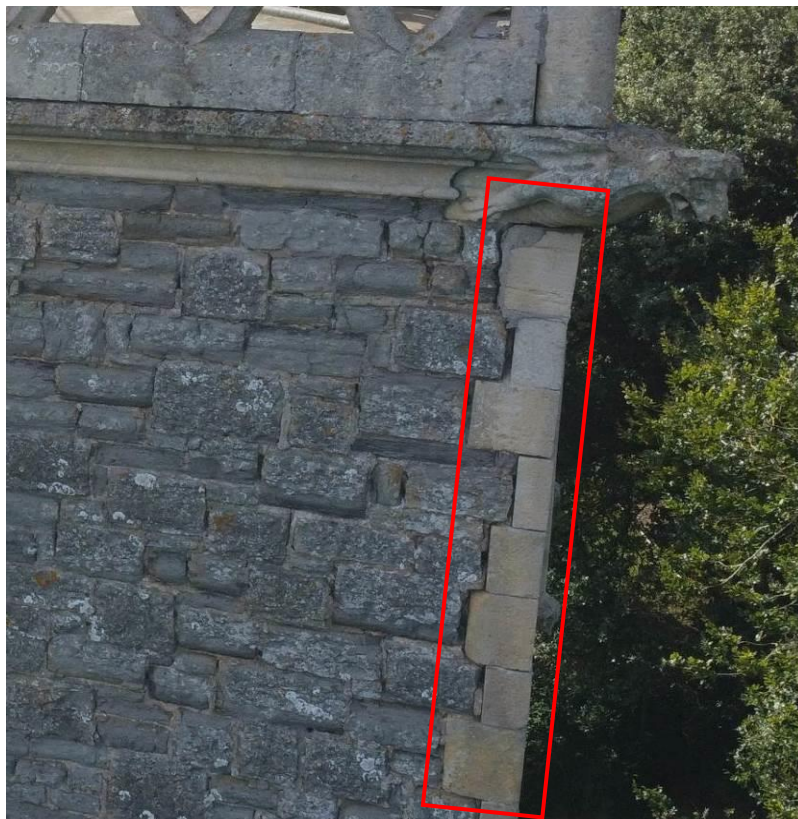
Figure 20 - DJI_0201 Displaced & Loose Quoins in North Elevation Belfry Level
