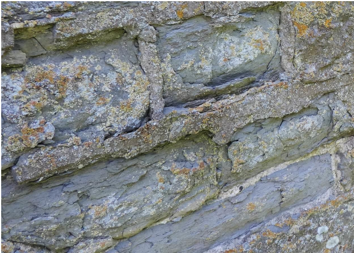
Figure 5 - P1000458 Example Area of Decaying Masonry Exacerbated by the Marine Environment and Cement Pointing in Tower West Elevation above West Window
