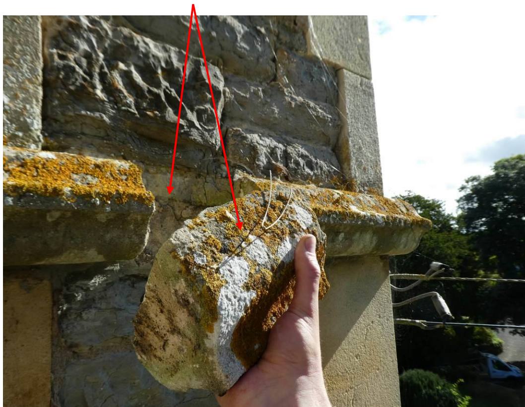
Figure 47 - P1000376SW Fractured Masonry Removed from Stair Turret South West Elevation 3 rd Stage String Course During Survey
