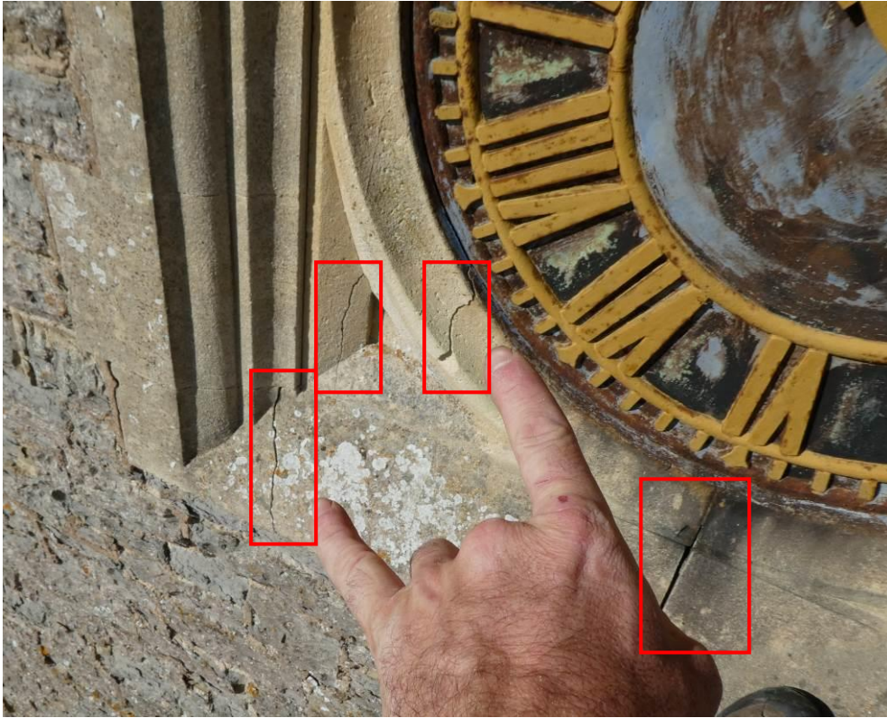
Figure 39 - P1000329 Fractures & Open Joints in East Elevation Clock Surround
