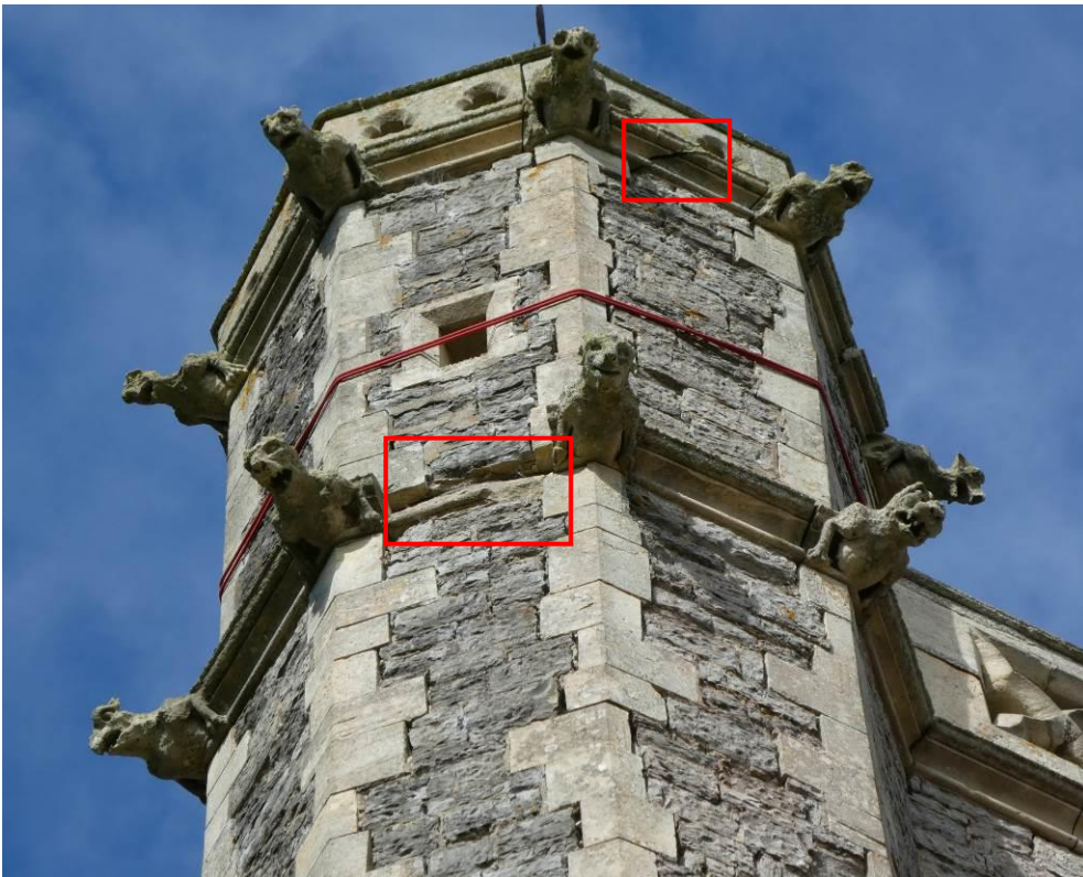
Figure 43 - P1000481 Masonry Fracture & Missing String Course Section in Stair Turret Tower East & South East Elevations
