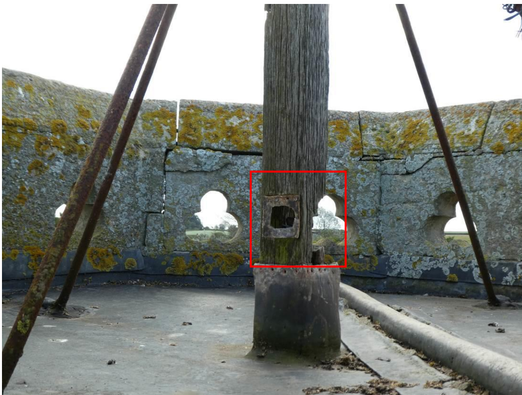
Figure 52 - P1000489 Rusting Weather Vane Stays & Severely Compromised Wooden Central Pole
