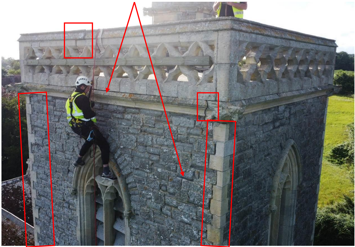
Figure 12 - DJI_0200a Severe Displacement of Parapet & Open Joints in Walls & Along Quoins
