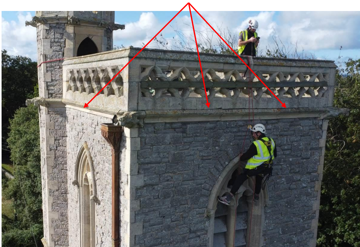
Figure 10 - DJI_0202 Masonry 'Jacking' & Displacement Visible in All Four Elevations of the Tower Parapet
