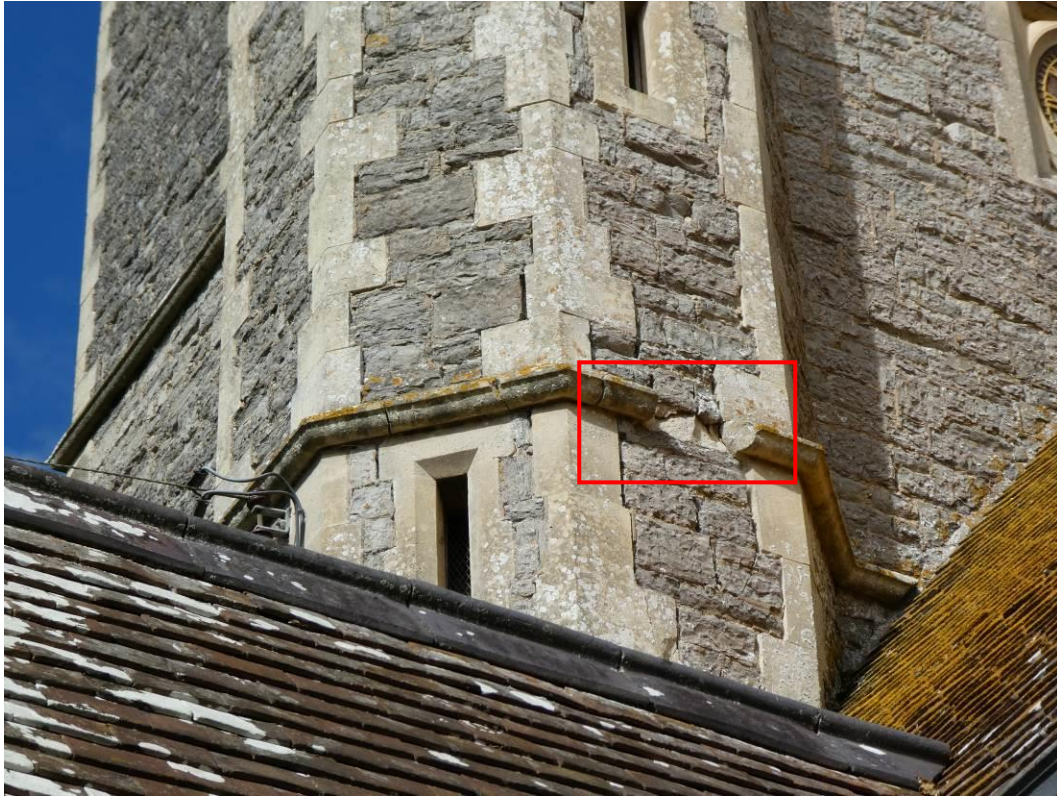
Figure 48 - P10000205 Missing 2nd Stage String Course Likely Resulting from Rusting Ring Beam in Stair Turret East Elevation
