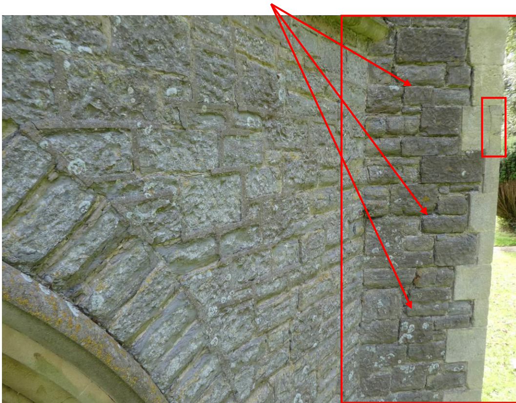
Figure 32 - P1000476 South West Buttress Appears to be Under Great Structural Stress
