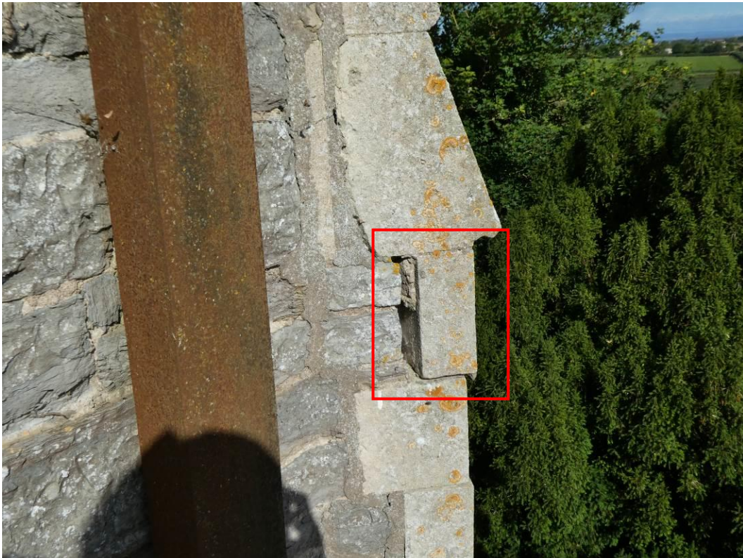
Figure 40 - P1000327 Unstable Quoin in East Elevation North East Buttress
