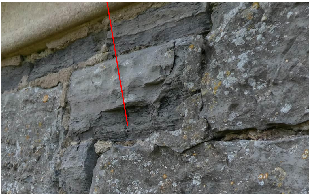
Figure 24 - P1000241 Example Lias Decay Where Mortar Repair Would Aid in Water Runoff
