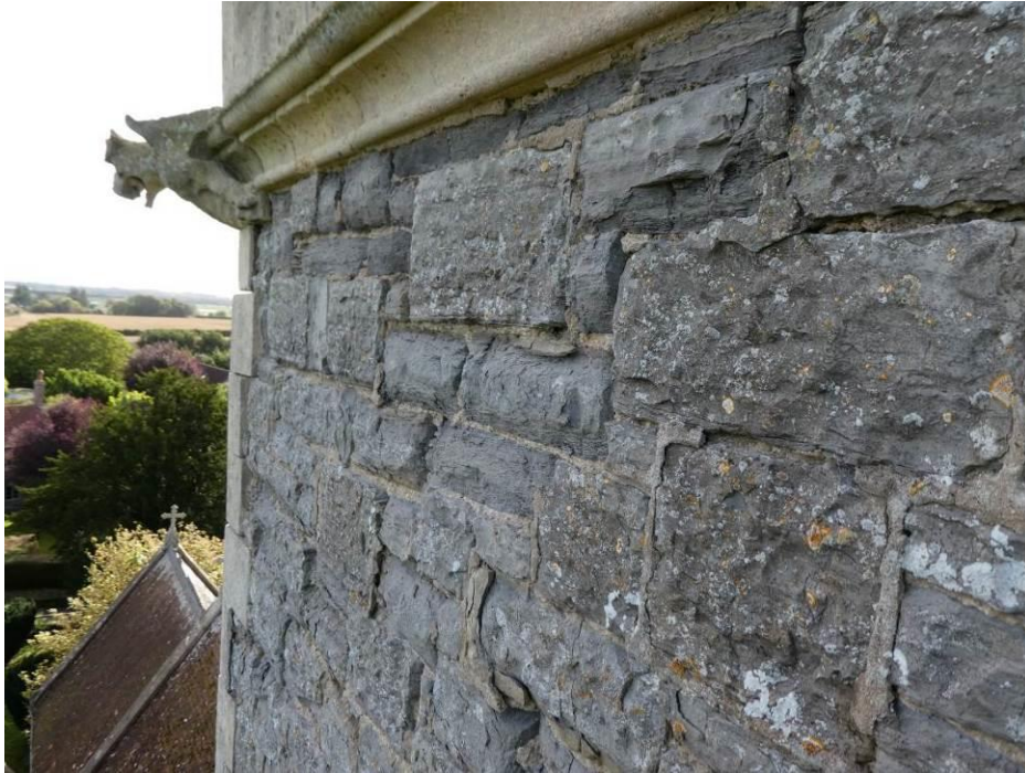
Figure 23 - P1000241 Example Area of Deteriorating Lias Masonry & Cement Pointing in North Elevation Belfry Wall
