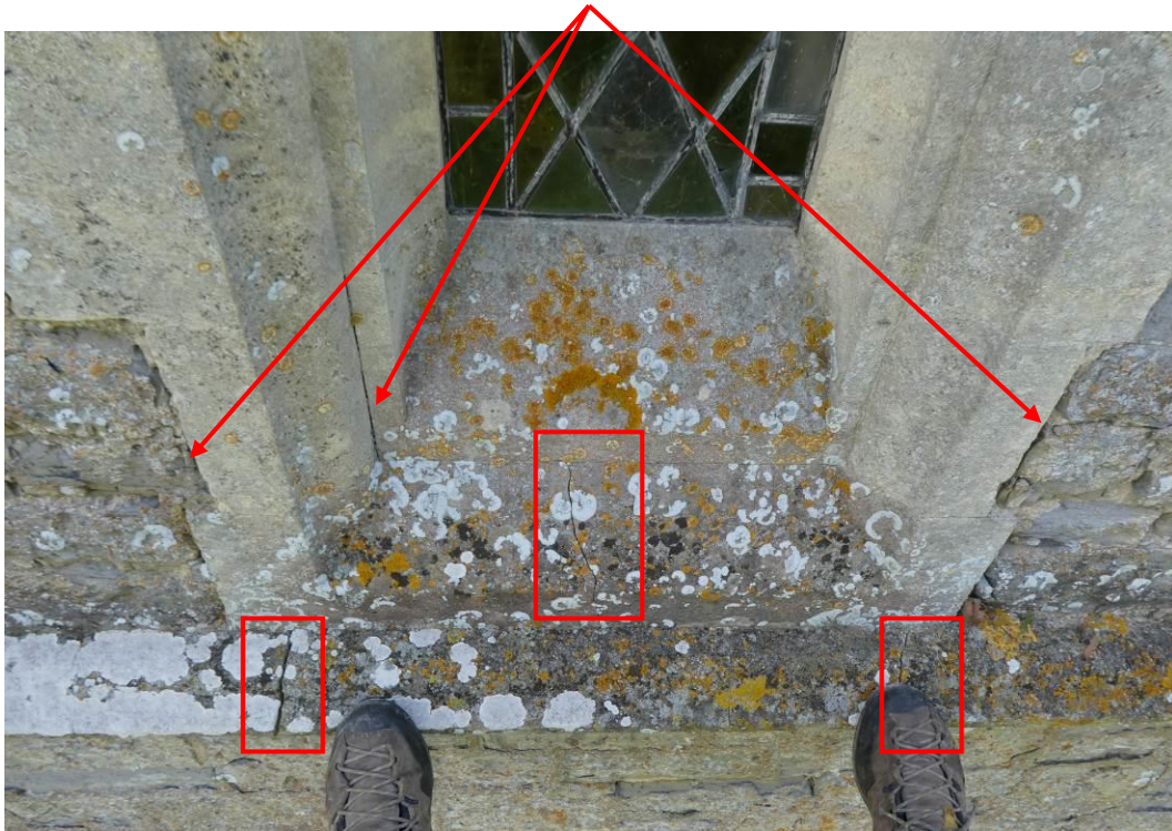
Figure 28 - P1000450 Masonry Fractures & Open Joints in 3rd Stage Window Sill & Reveals West Elevation
