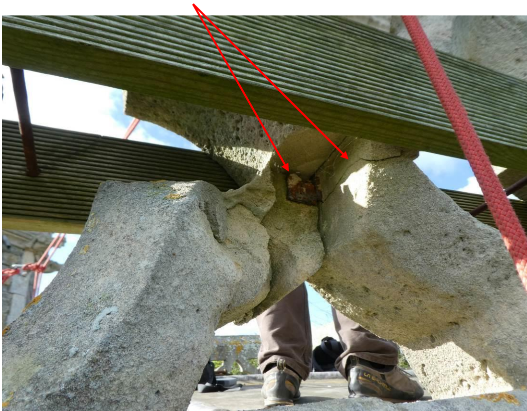
Figure 14 - P1000239 Example Rusting Fixing & Associated Masonry Fractures in North Elevation Parapet
