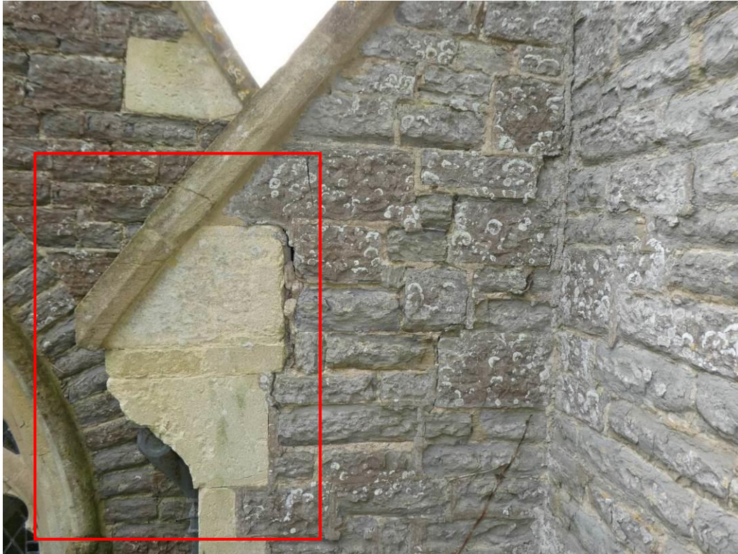
Figure 21 - Precarious Kneeler Stone in North East Buttress 2nd Level
