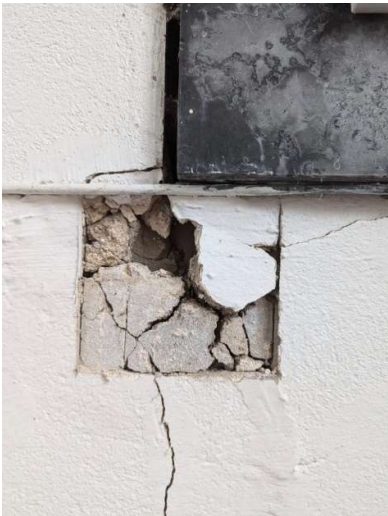
Figure 20 Partial removal of the topcoat plaster beneath the monument, revealing the fragmented second coat of plaster beneath
