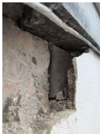
Figure 23 The plaster appears to have detached from the brickwork
