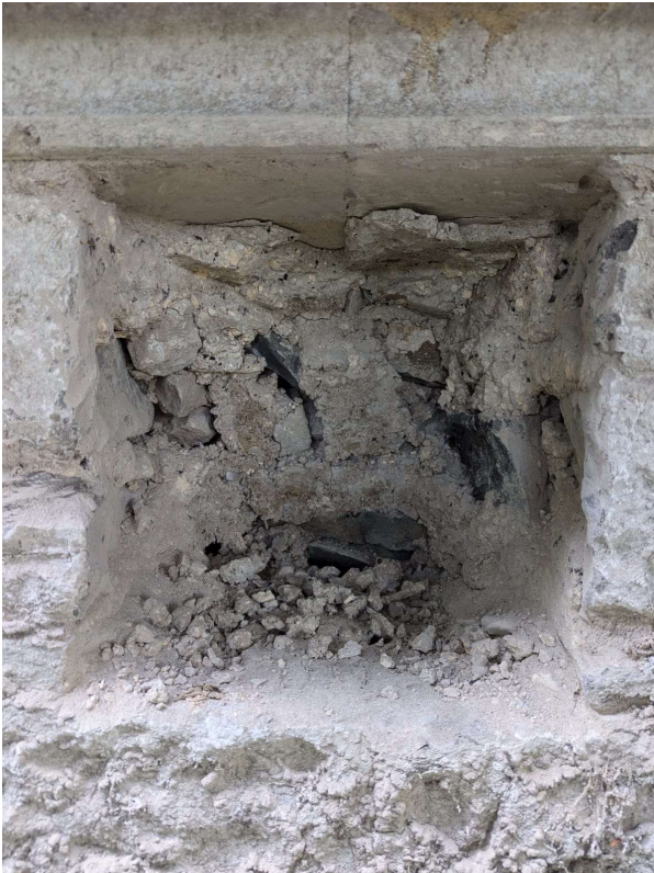
Figure 7 The void with both stones removed and original bedding and pointing mortar visible
