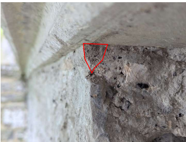
Figure 9 The pinkish mortar found on the face of the joints is indicated in red
