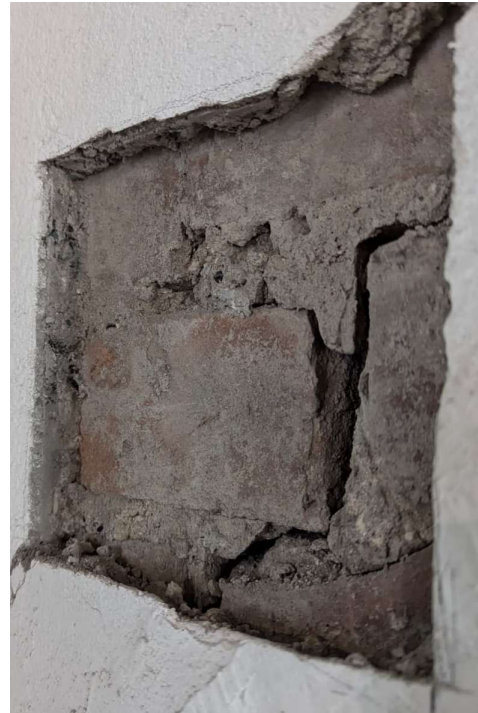
Figure 19 Detail of cracking through the joints of the brickwork
