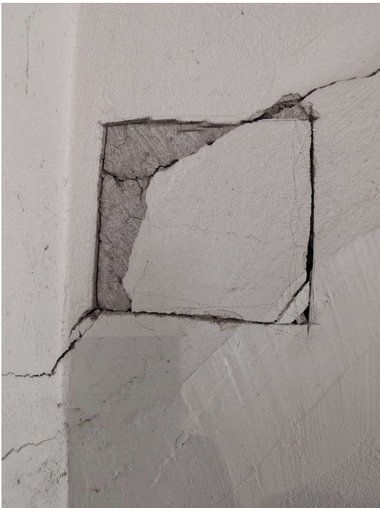
Figure 16 The window with an area of topcoat plaster removed
