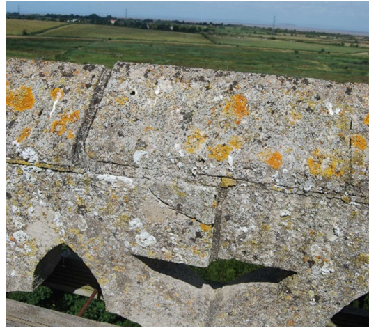
Figure 20 Fractured corner and displacement to the central panel on the north elevation.
