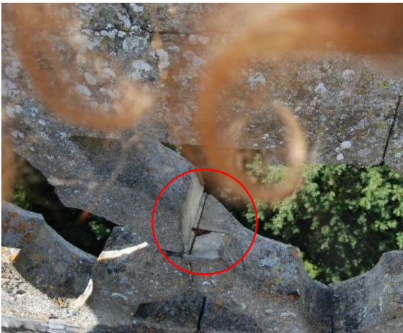
Figure 17 Corroded iron fixing visible in the lower bed at the centre of the broken panel to the north west corner (west elevation).
