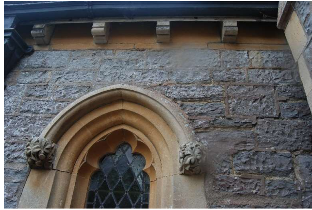
Figure 31 Failing cement pointing above the south porch east window.
