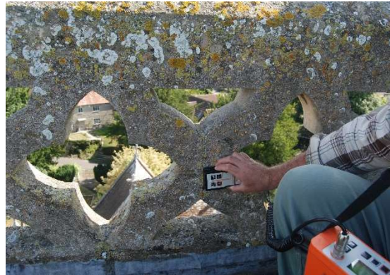
Figure 16 Example of an iron fixing detected at the centre of a panel on the east elevation. It is assumed that all panels contain similar central iron fixings.
