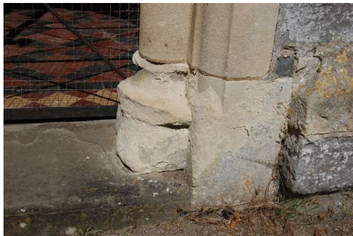
Figure 42 Surface blistering and loss to the lower east jamb
