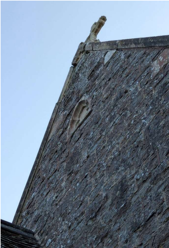
Figure 64 Bulging of the vestry gable, open joints and leaning apex cross.
