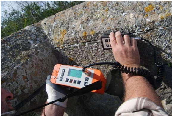
Figure 15 Opening up of the coping stone joint in the south west corner (west elevation), and detection of iron fixing in this location.
