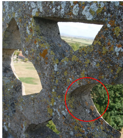
Figure 18 Sealed slot on the inside of a panel at the north east corner (east elevation). It is assumed that the iron fixings have been installed this way throughout the parapet.
