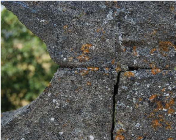
Figure 19 Example of displacement caused by embedded metal fixing at the central joints of a panel.
