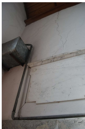
Figure 9 Vertical cracking to the west wall of the south chapel/organ chamber
