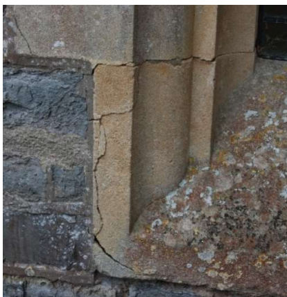
Figure 36 Detail of cracking to the external lower south jamb/cill. Cement pointing visible.
