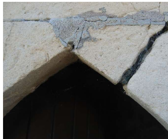
Figure 25 Large crack, visible pin and cement pointing to the vice turret door head.
