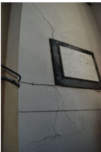
Figure 8 Vertical cracking to the east wall of the south chapel/organ chamber
