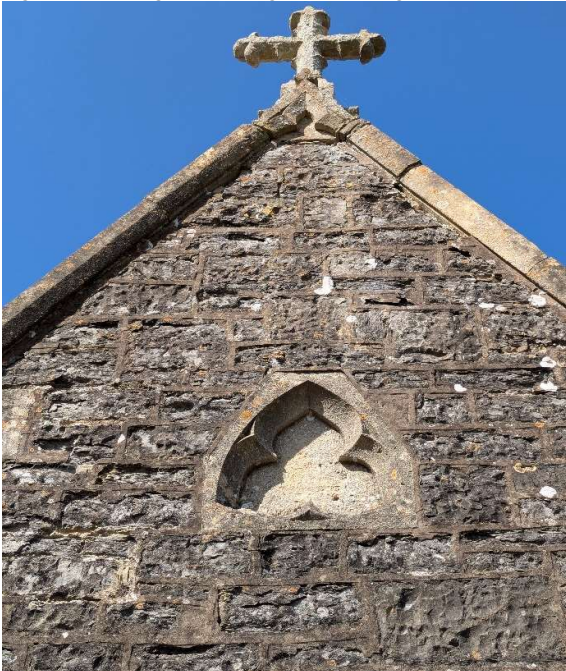
Figure 54 Open joints and movement to the gable copings
