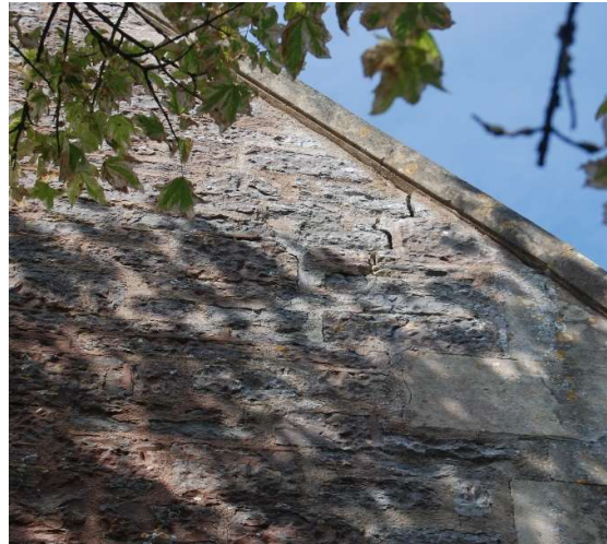
Figure 59 Cracking through upper north corner of the chancel east gable
