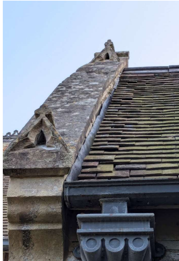
Figure 65 Point of water ingress where lead flashing is open behind the vestry gable
