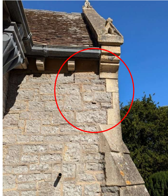
Figure 55 Stress crack to the gable on the west elevation
