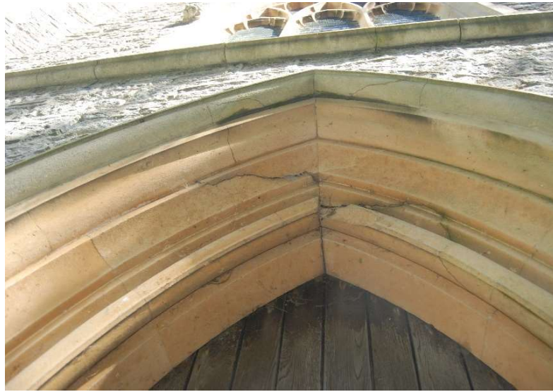
Figure 77 Cracking over the tower west door
