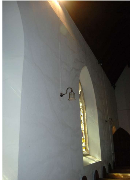
Figure 7 Lateral crack along the south nave wall at upper level. Stretch marks and historic plaster patching visible.
