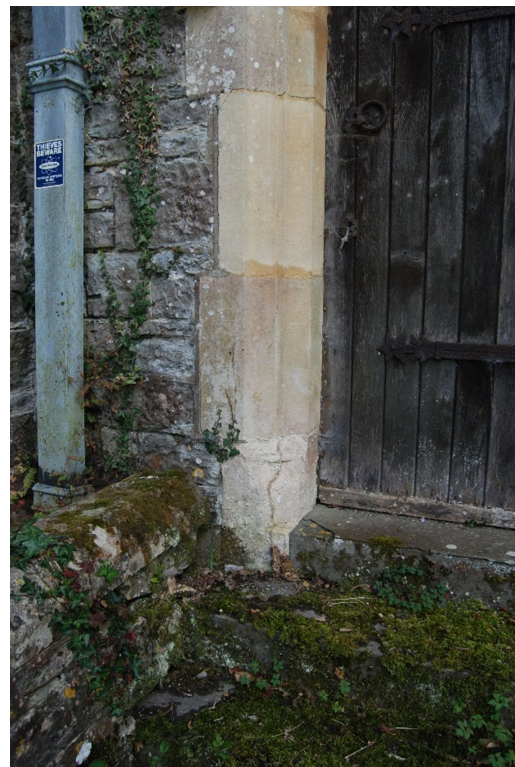
Figure 63 Evidence of damp at the base of the vestry east door and around the base of the downpipe
