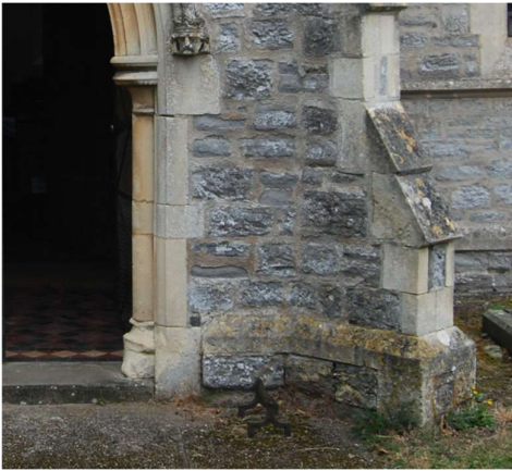
Figure 30 Lower east side of south porch door with cement pointing, weathered faces of blue lias and open joints to the buttress visible.
