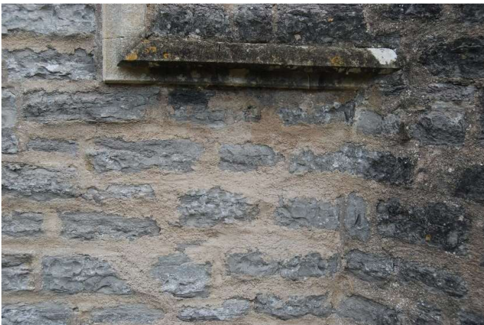
Figure 61 Detail of smeared cement pointing to the blue lias beneath the string course of the east chancel
