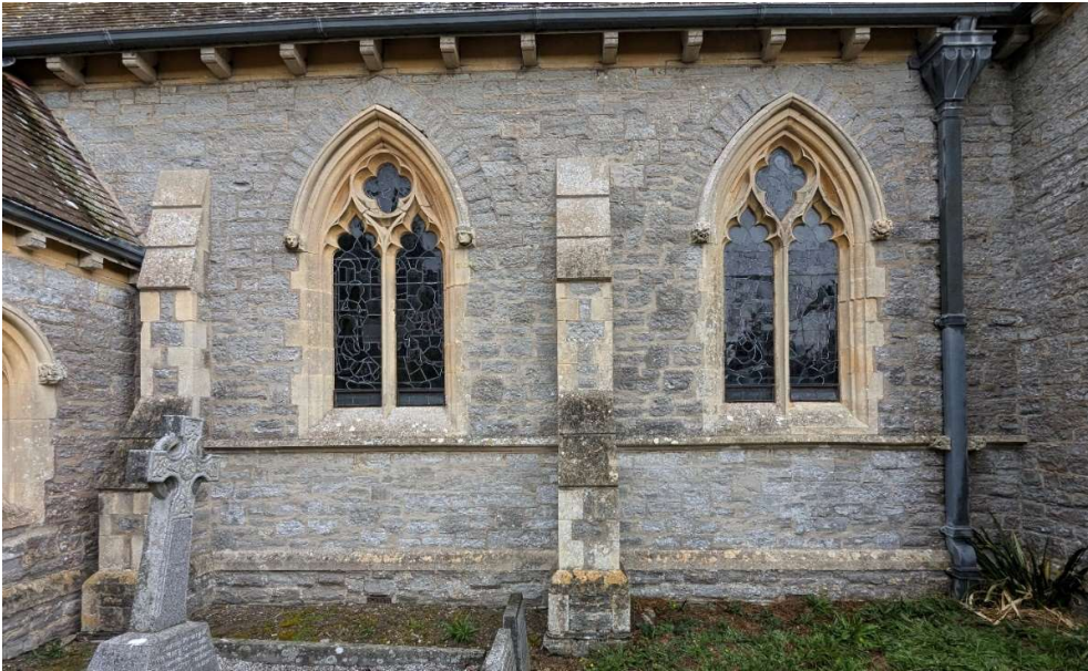
Figure 43 South nave wall showing dipping of the string course to either side of south windows 1 and 2.
