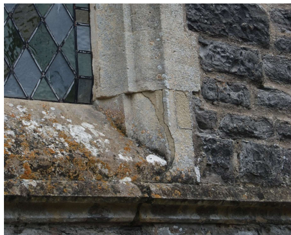
Figure 52 Cracking to the lower east corner at cill level
