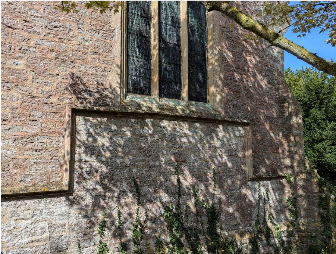
Figure 57 Chancel east end showing variation in stone colour beneath the undulating string course. Cement pointing throughout.
