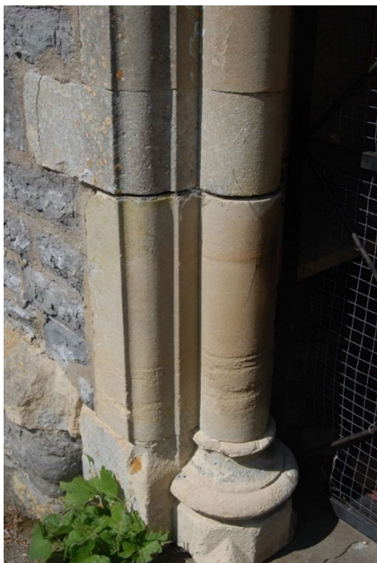
Figure 41 Displacement and open joints to lower west jamb
