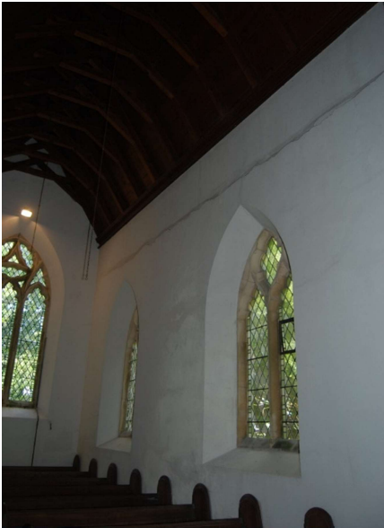
Figure 6 Lateral crack along the north nave wall at upper level.
