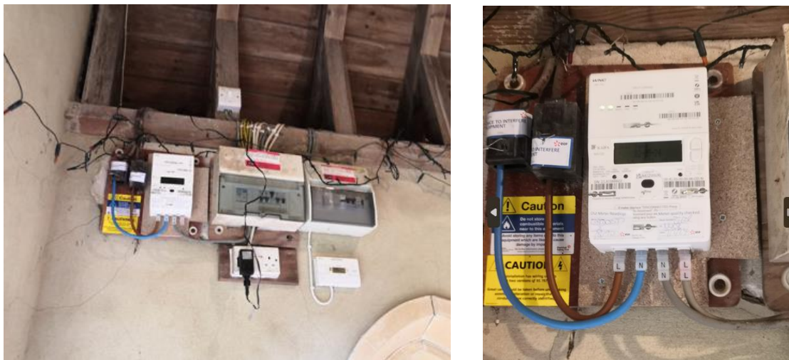
Existing electrical cutout, meter and distribution board
