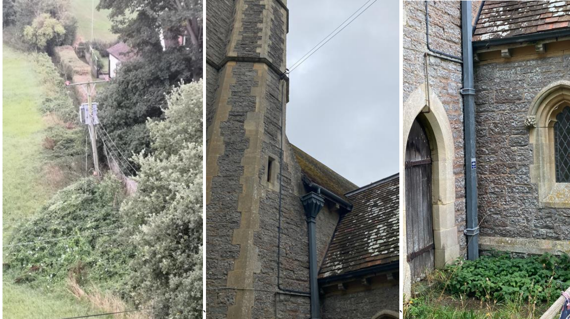
Incoming electrical supply from transformer in neighbouring field entering into the porch
