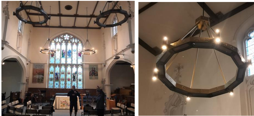
HALO Infra-red Heaters installed at St. Matthew's, Cotham, Bristol, with integrated up/down LED lighting above altar.
