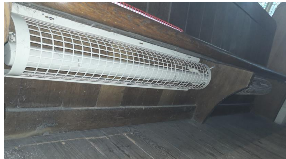
Existing Under Pew Heaters
