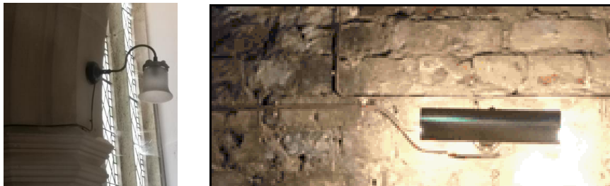
Existing gas lamps and microbore gas pipework at St. Mary Magdalene (left), MF example of MICC cabled heritage lighting.
