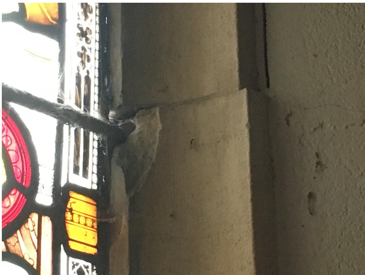
Expanding tie bar spalling stone work. It is likely that the misalignment of the jamb is due to other factors.
