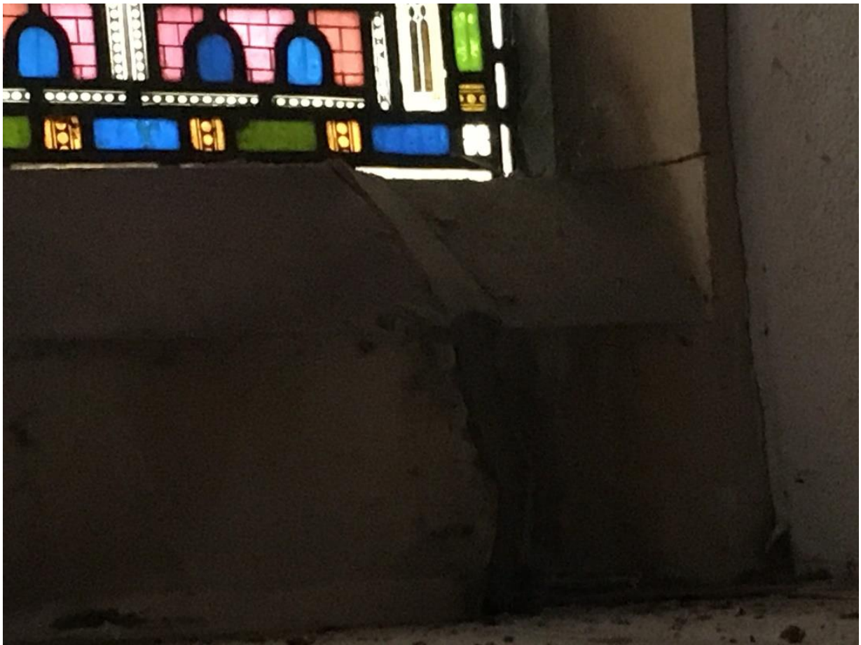
Misaligned sill block
