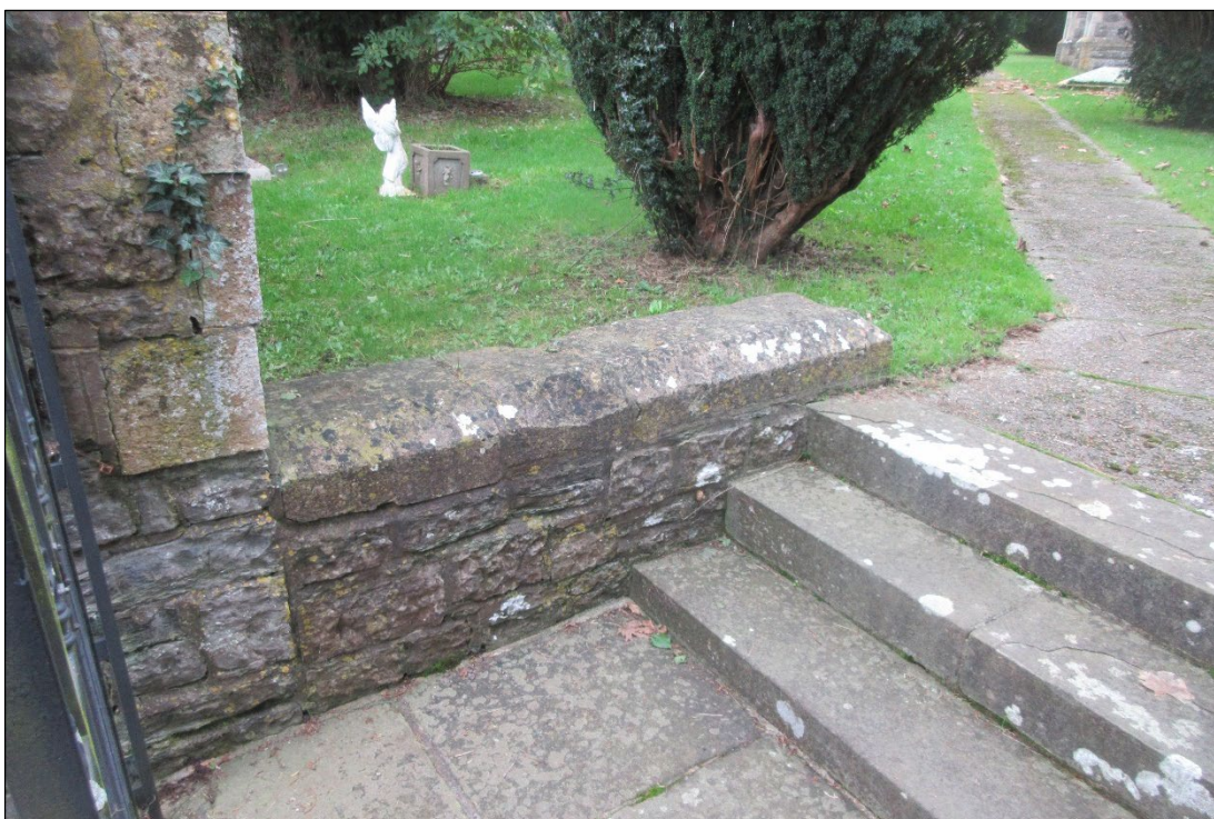
There is no handrail to assist with access up the steps.
