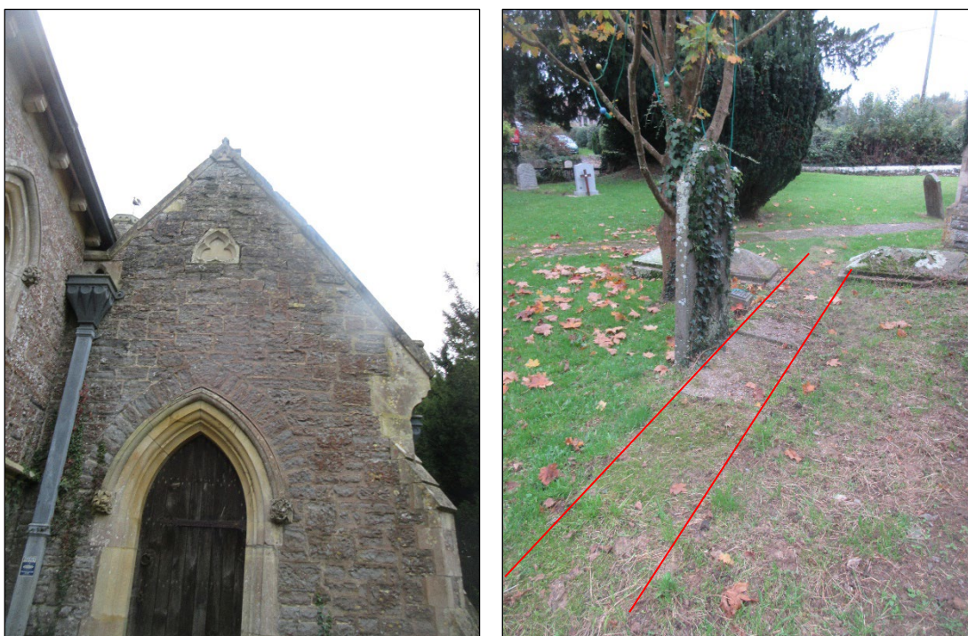
Above: The wall above the vestry door and the existing overgrown concrete path.
