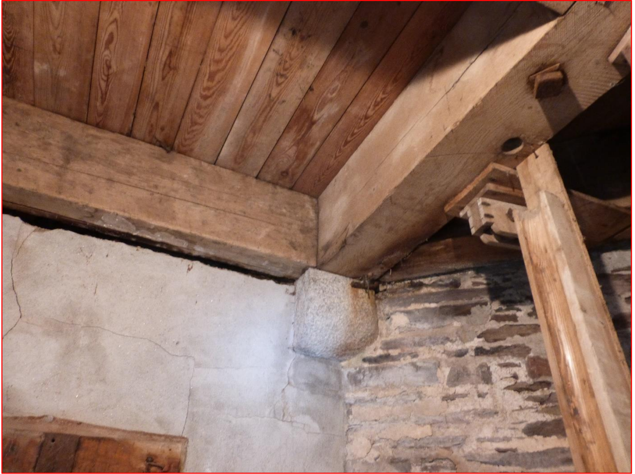
Photo: The bellframe foundations and belfry floor at Revelstoke (Noss Mayo) Devon as installed by John Warner in 1881
