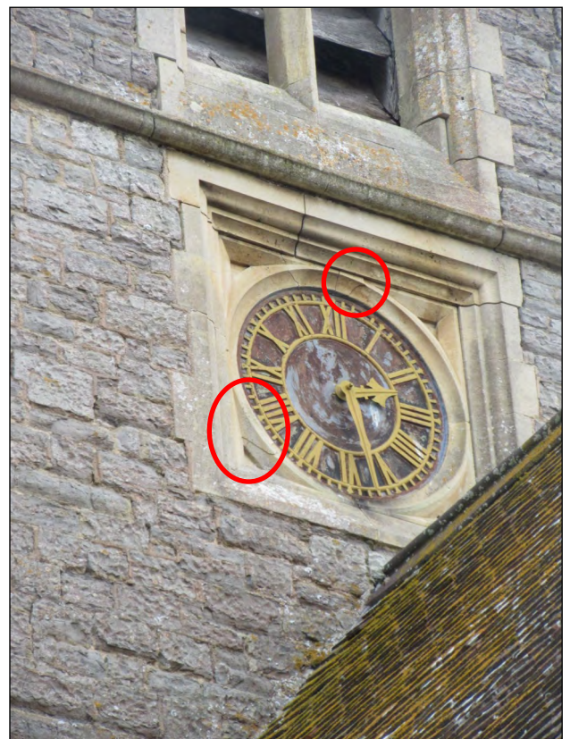
046 Damage to the clock dial surround probably as a result of iron cramps.
