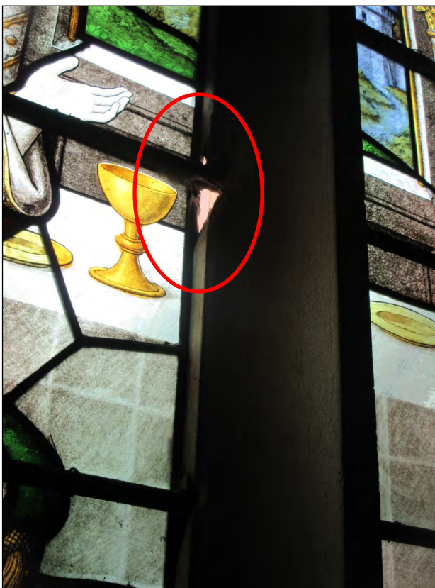
026 Damage to stonework caused by the decay of a tie bar — Window sV.
