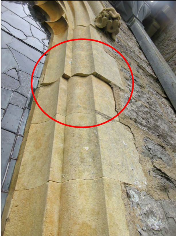
024 Disturbed masonry to Window sIV.
