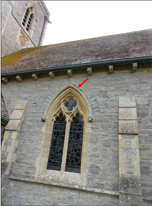
017 The open joint above the hood mould to the windows.
