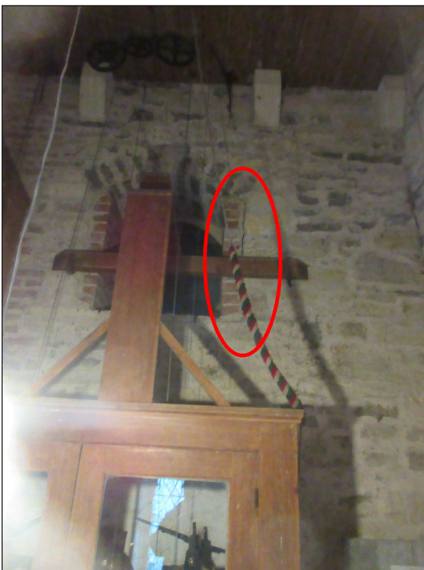
041 The detaching brick lining to the reveal of the east window in the tower.
