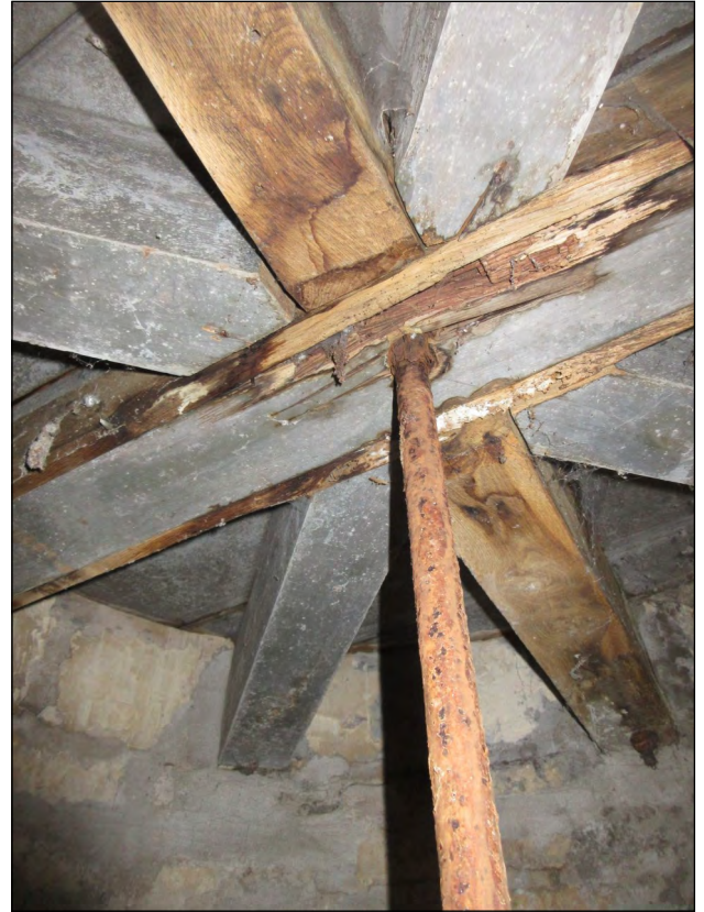
033 Timber decay to the underside of the vice turret roof.
