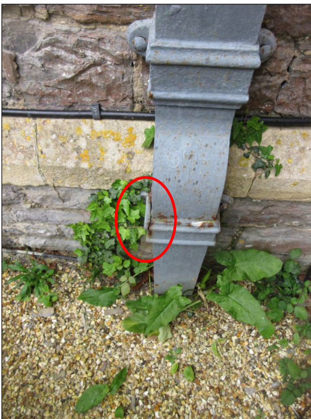
011 A fractured collar to the downpipe.
