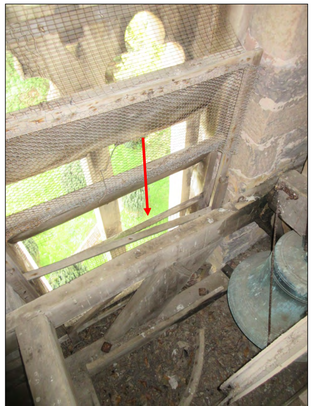
042 Tower louvre decay and open access for jack-daws.
