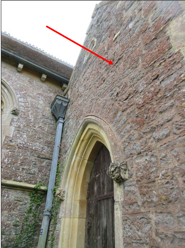
020 The bulging east gable of the vestry.
