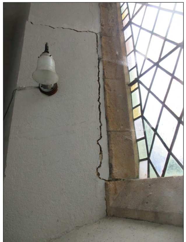
023 Cracking to the South Chapel window east reveal.
