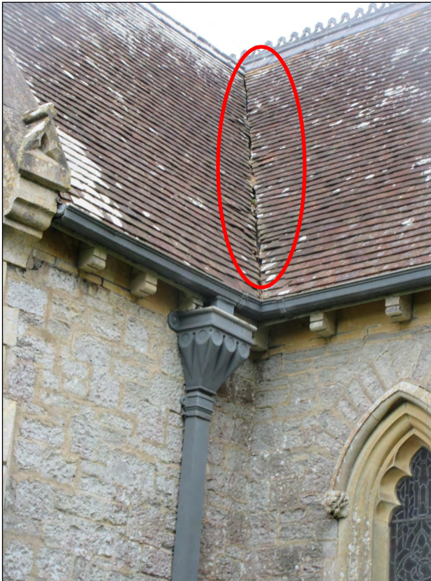
001 Disturbed slates in the valley between the chancel and South Chapel
