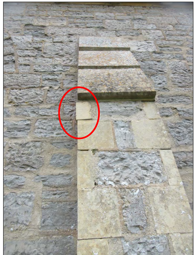
016 A typical disturbed quoin.
