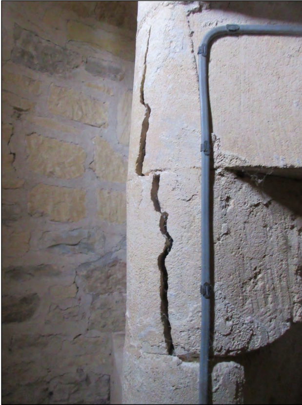
032 The cracking to the vice turret stair newel.
