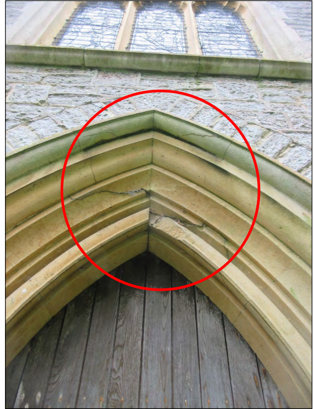
029 Masonry damage to the head of the west door.
