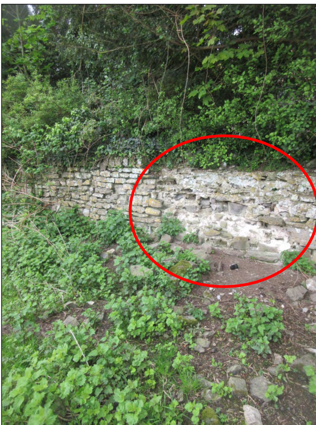
049 The loss of wall face to the north facing churchyard wall.
