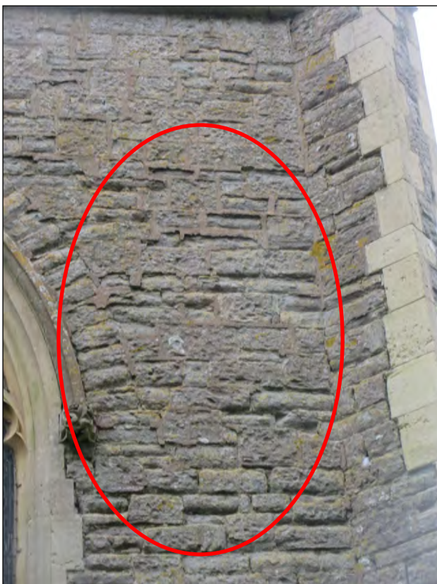
045 Cement pointing to the tower is causing accelerated decay of the stonework.
