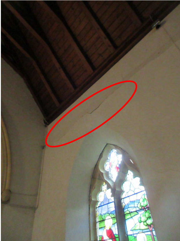
051 The horizontal cracking to the nave plaster.
