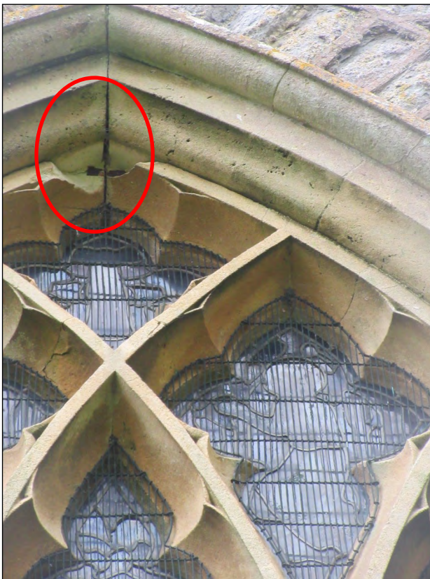
030 Iron cramp damage to the head of the west window.
