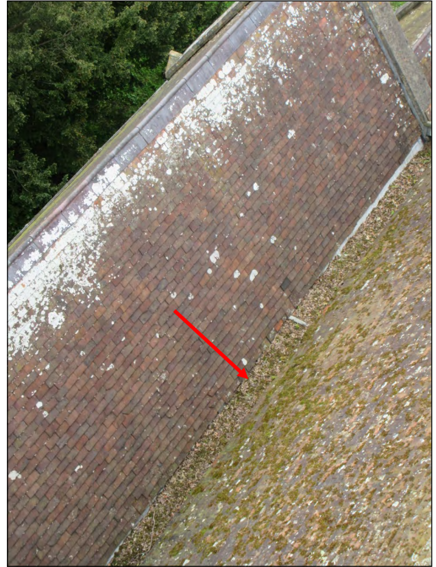
006 The central valley needs clearing.
