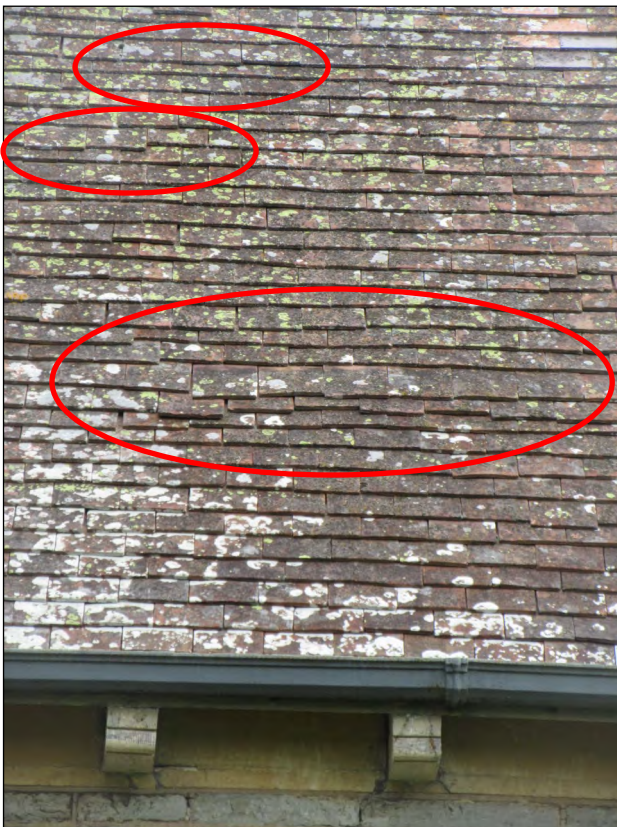
007 Slipped tiles on the nave roof are indicative of nail batten fixing failure.
