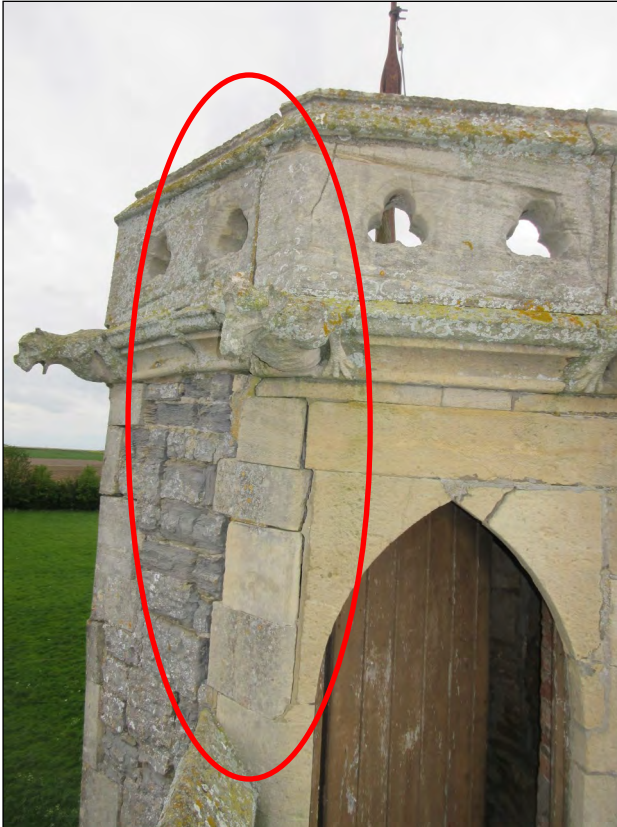
035 Very disturbed stonework at the top of the vice turret.
