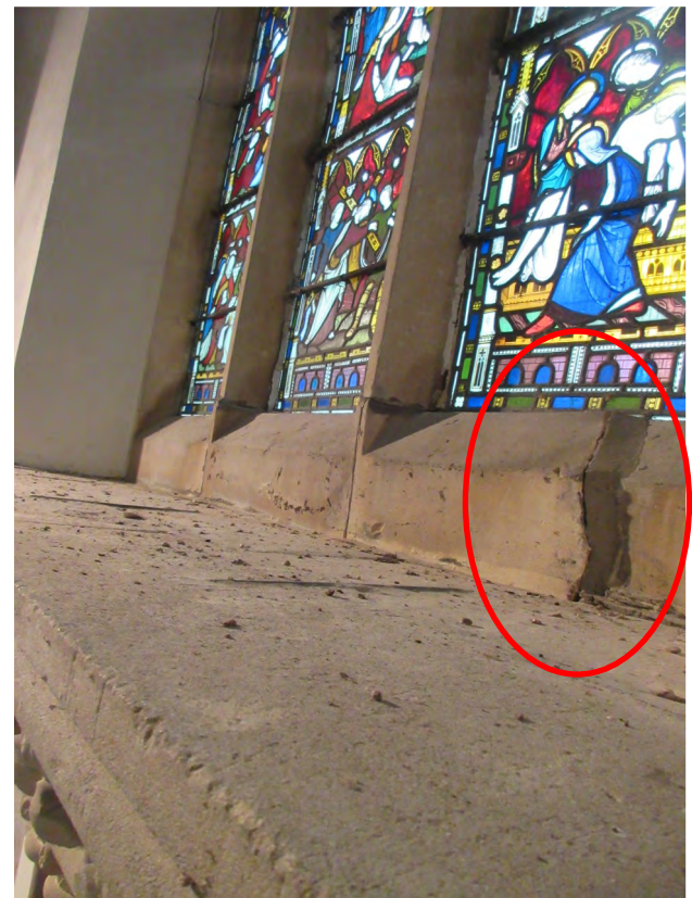
054 Displaced and misaligned stonework to east window is longstanding and appears to be stable.
