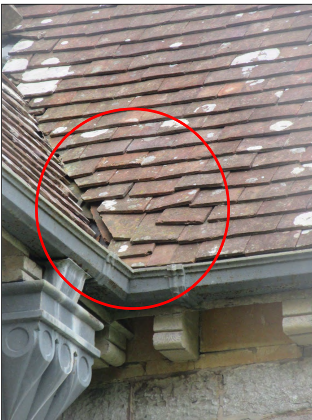
003 Disturbed tiles at the base of the west slope of the South Chapel roof.
