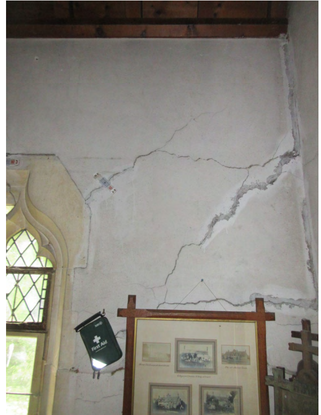
052 Plaster cracking in the vestry.
