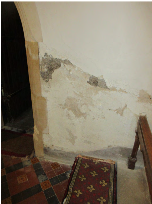
053 Decaying plasterwork at low level on the north wall of the chancel.
