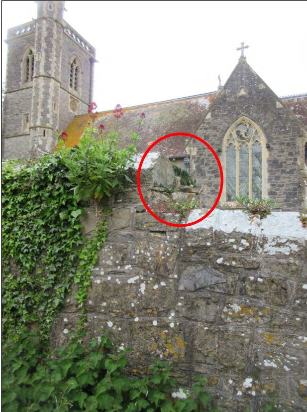
047 A missing section of churchyard wall capping.
