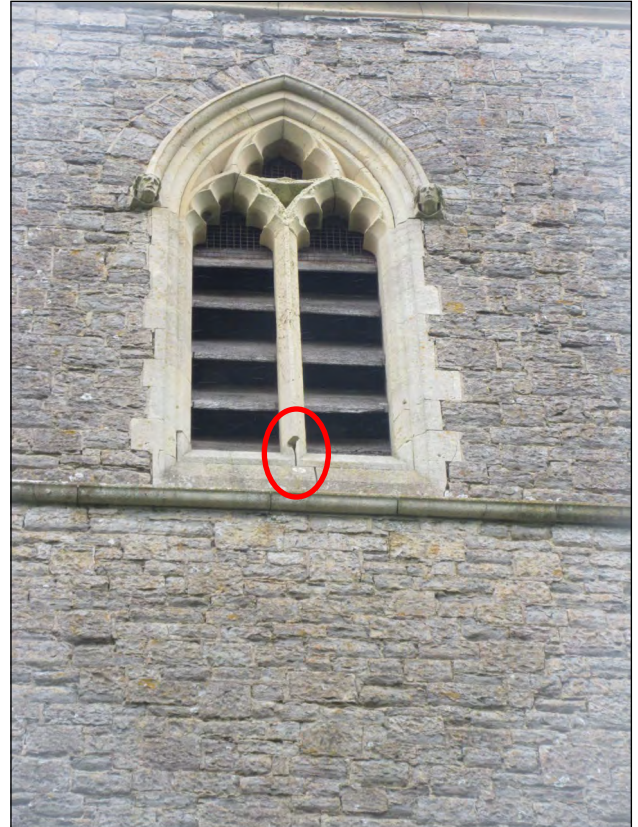
044 Possible iron cramp damage to the west window.
