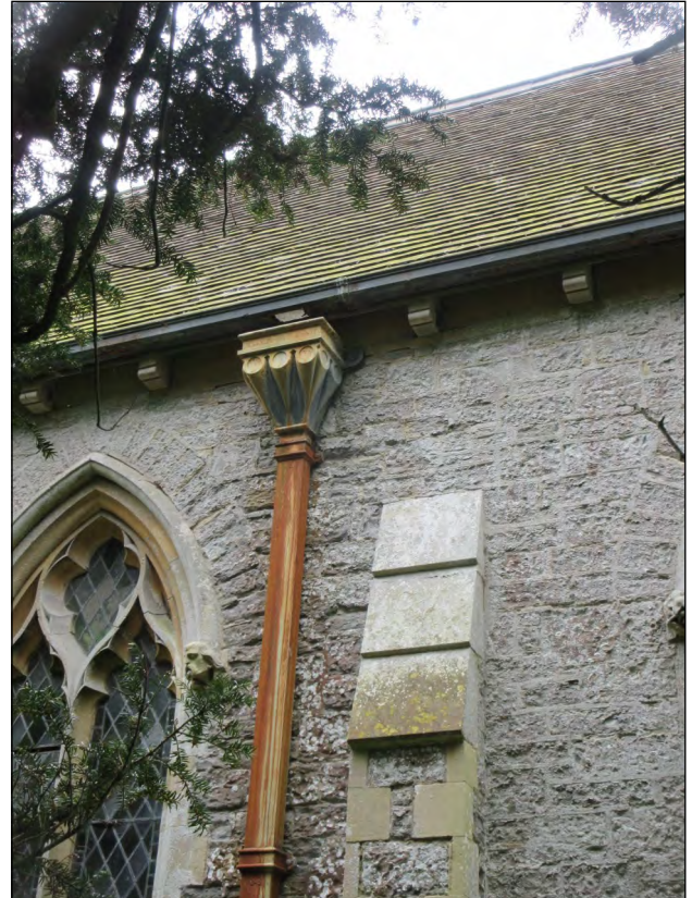
010 Rust staining caused by a blockage in the downpipe.
