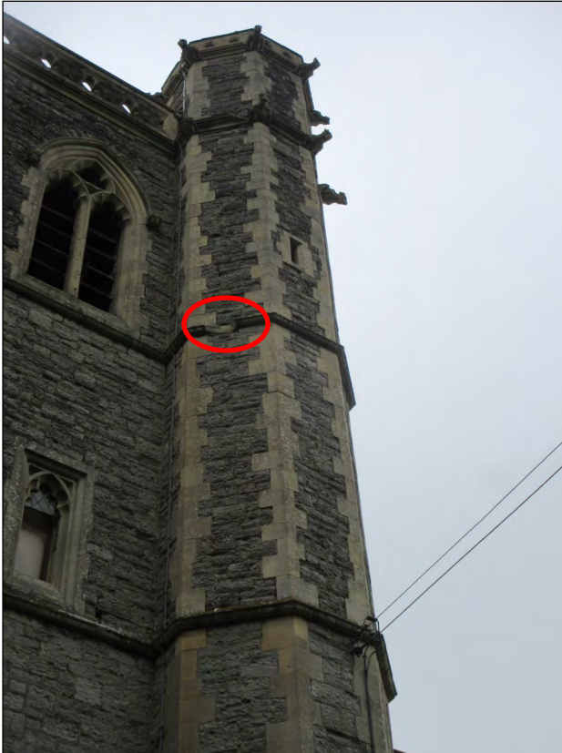
043 A missing section of string course from the vice turret.
