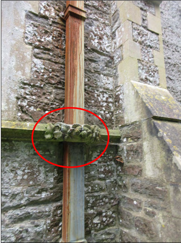
013 The last remaining downpipe collar.
