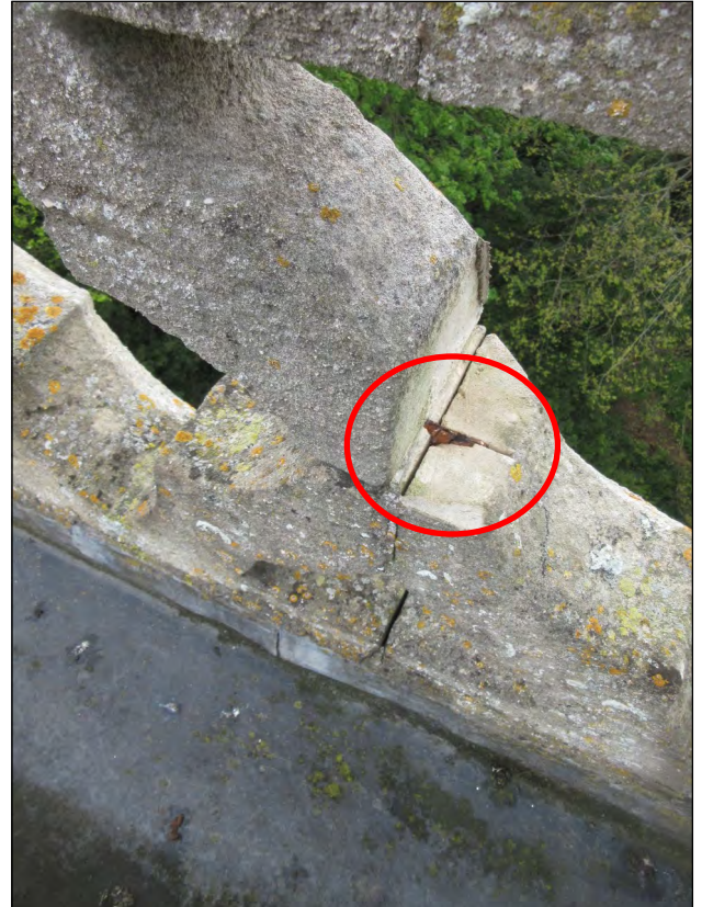
040 Decaying cramps in the tower parapet stonework.
