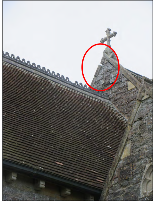
014 Open joints in the chancel arch coping.
