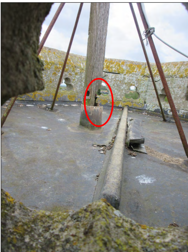
037 Decay to the base of the vice turret weathercock post.
