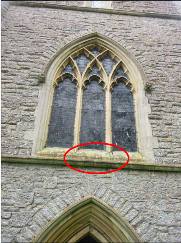
028 Open joints in the cill of the west window.
