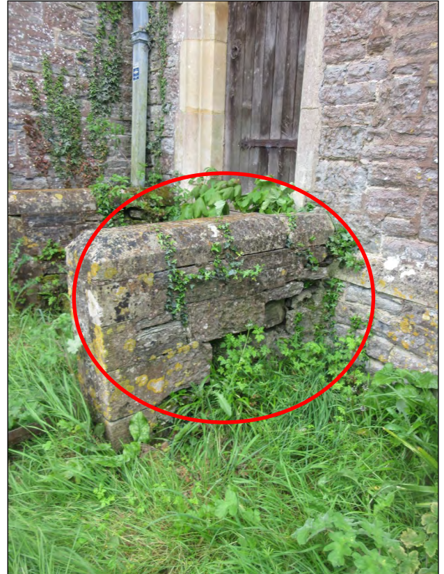
021 The flanking walls to the vestry steps need to be rebuilt.
