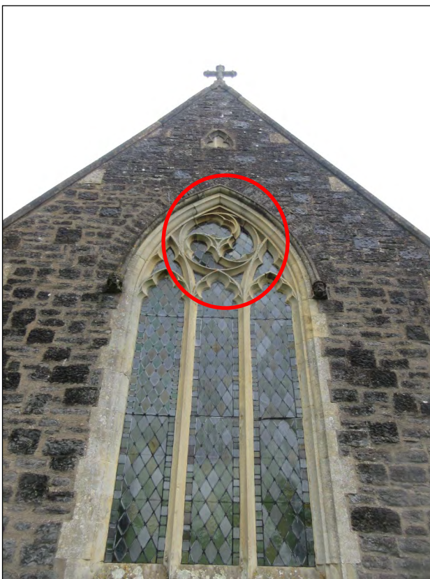
022 The disturbed tracery stonework and glass of the South Chapel window.
