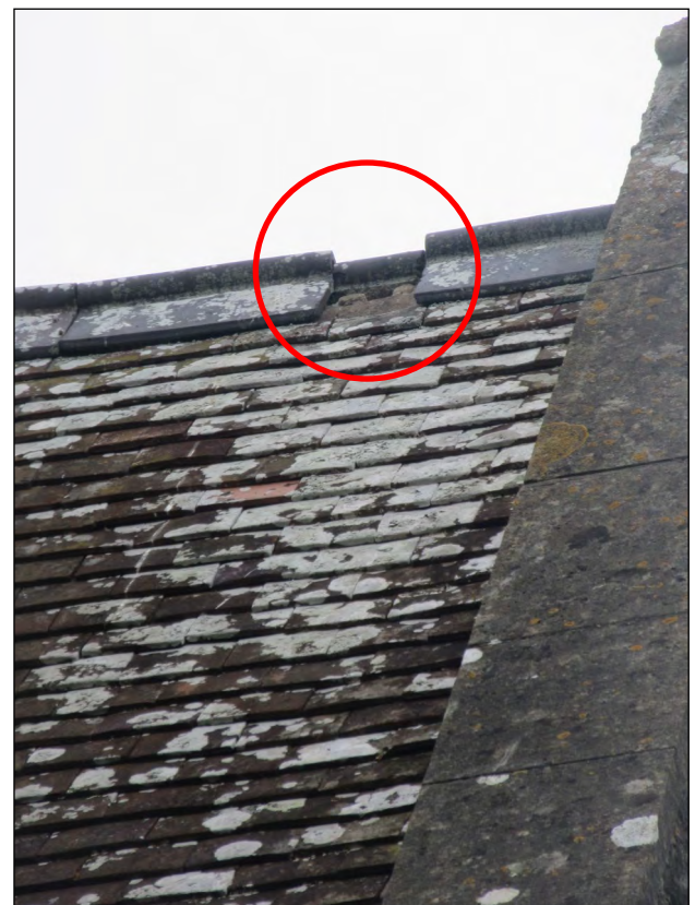
004 A damaged ridge tile on the South Chapel roof.
