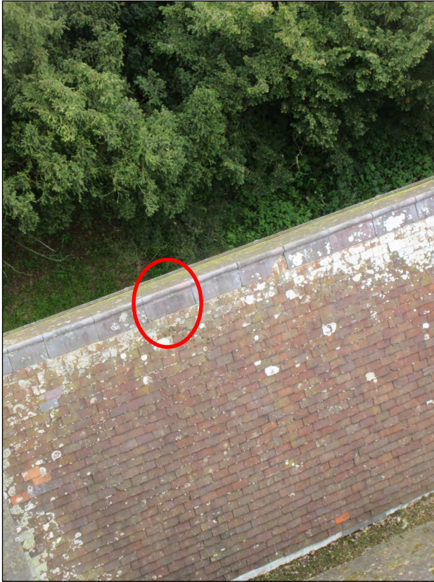
005 A cracked ridge tile on the north aisle roof.
