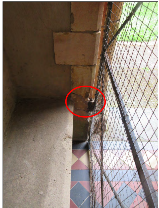
031 Pintel damage to the stonework of the South Porch gates.
