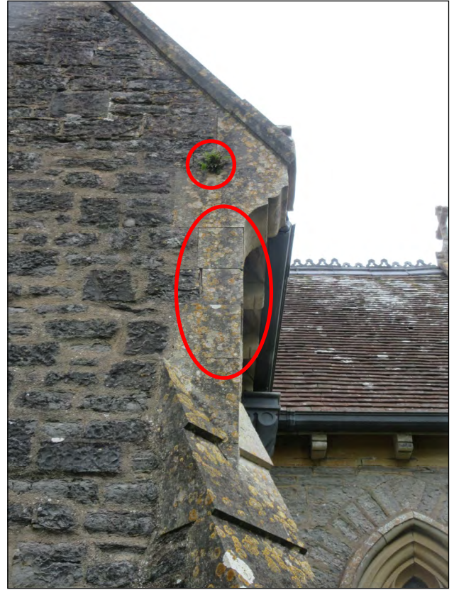
018 Disturbed quoins on the South Chapel. Vegetation above needs to be removed.
