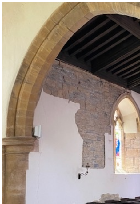
Photo 11 – Fracturing of South Aisle south wall adjacent intersection with South Transept.
