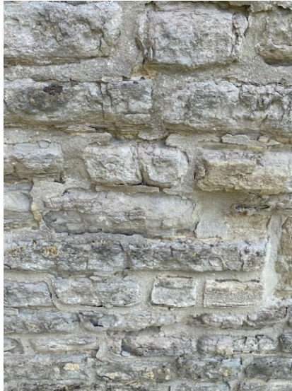
Photo 5 – Failure of cementitious face pointing and degradation of stonework.
