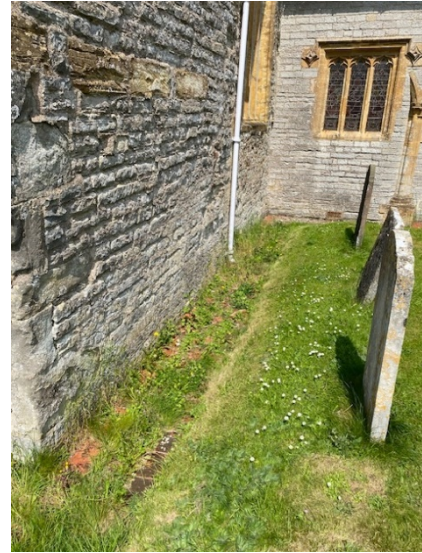
Photo 6 – Fractured / displaced drainage channel to perimeter of church
