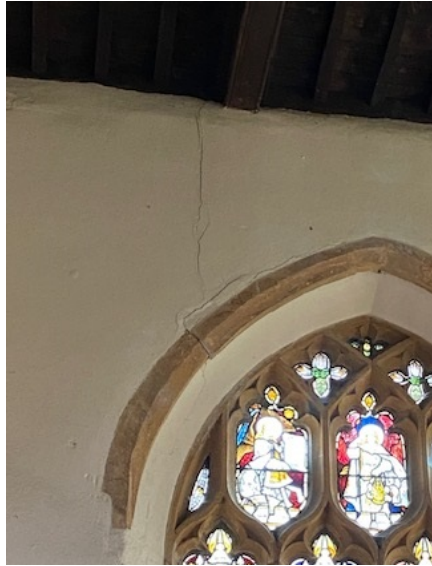
Photo 9 – Fracturing of East Window of South Transept with displacement of Voussoir.
