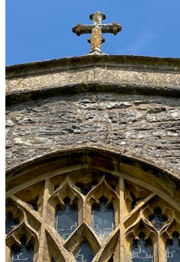
Photo 2 – Fracturing above head of window and displacement of window tracery
