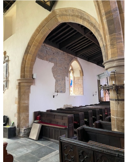
Photo 10 – Fracturing of South Aisle south wall adjacent intersection with South Transept.
