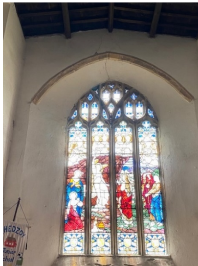
Photo 3 – South Transept, south window (internal view). Fracture through head of window extending down east reveal.
