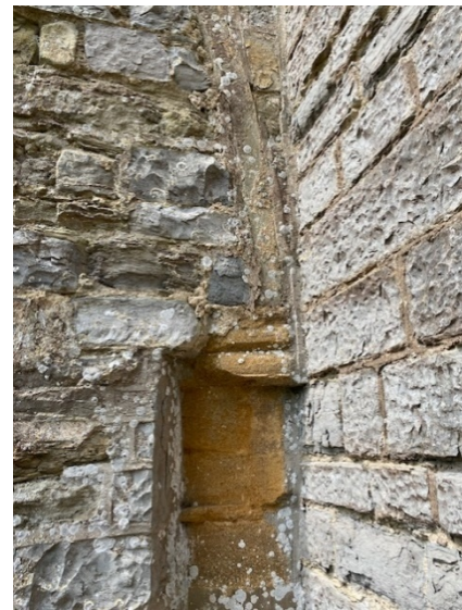
Photo 8 – East elevation of South Transept. Column and arch relating to earlier layout.
