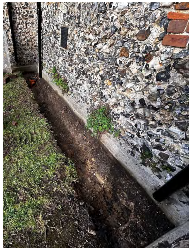
Plate 8b. Detailed view looking northeast along the line of Trench 3 showing C.19th concrete foundation addition.
