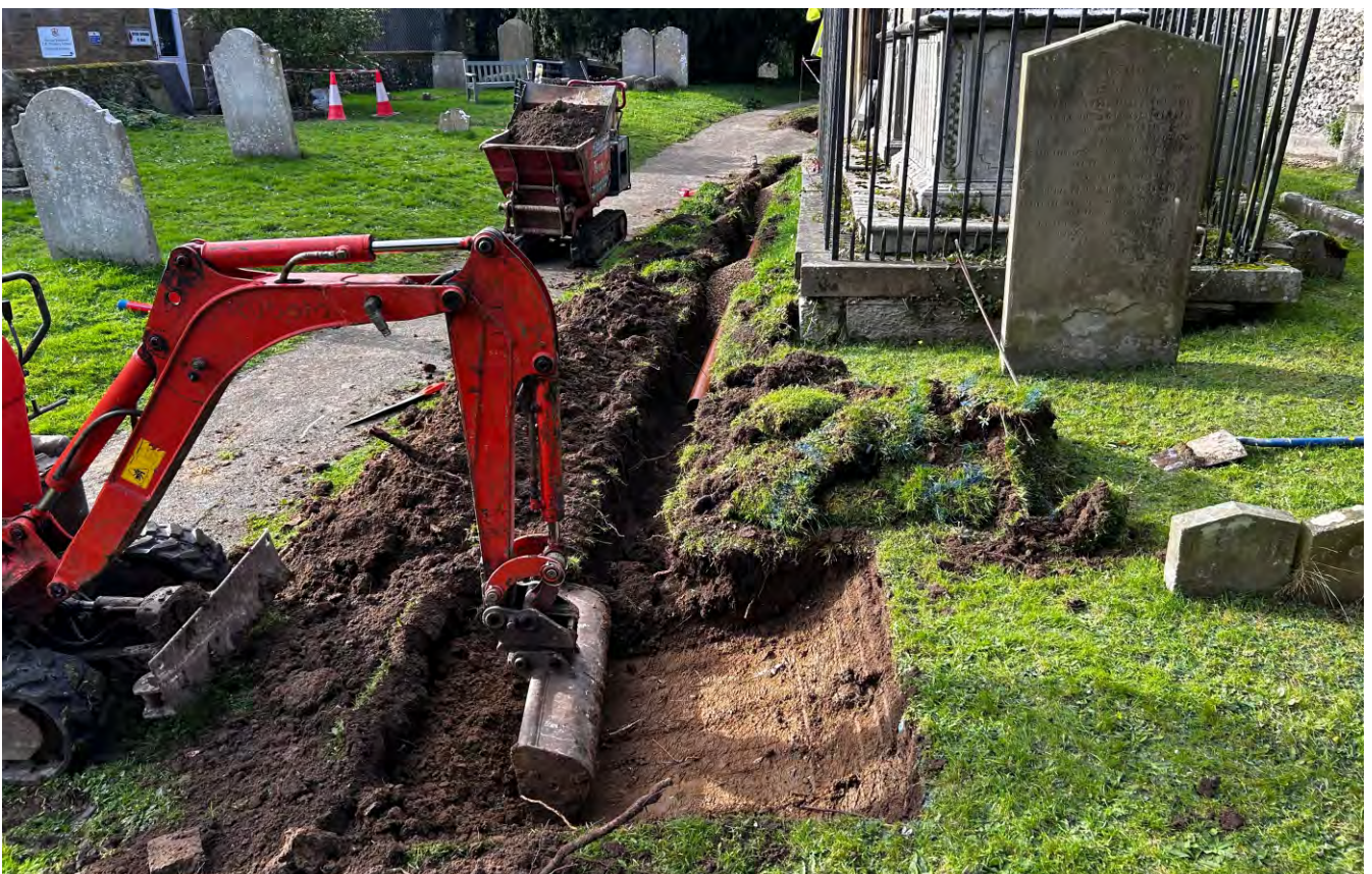
Plate 12. General view looking west along the line of Trench 4 showing Soakaway 2 being excavated adjacent the churchyard footpath.
