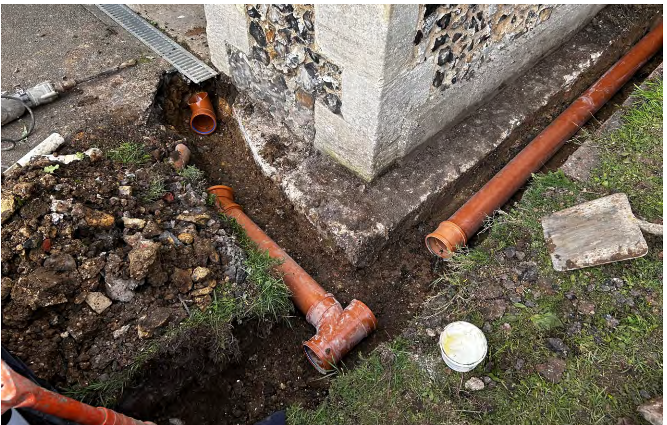
Plate 10. Detailed view looking northwest showing the southern end of Trench 3 connecting with the slotted drain across the threshold of the South porch door (top left) and continuing south to adjoin with the western end of Trench 4 ( note: concrete addition to porch's eastern wall foundation extending along the base of its southern front wall also ).
