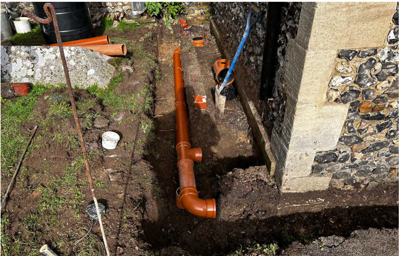
Plate 6. Detailed view looking north along the line of Trench 2 showing its route through the grassed area adjacent the existing 'french drain' with connections to existing rainwater down pipes..
