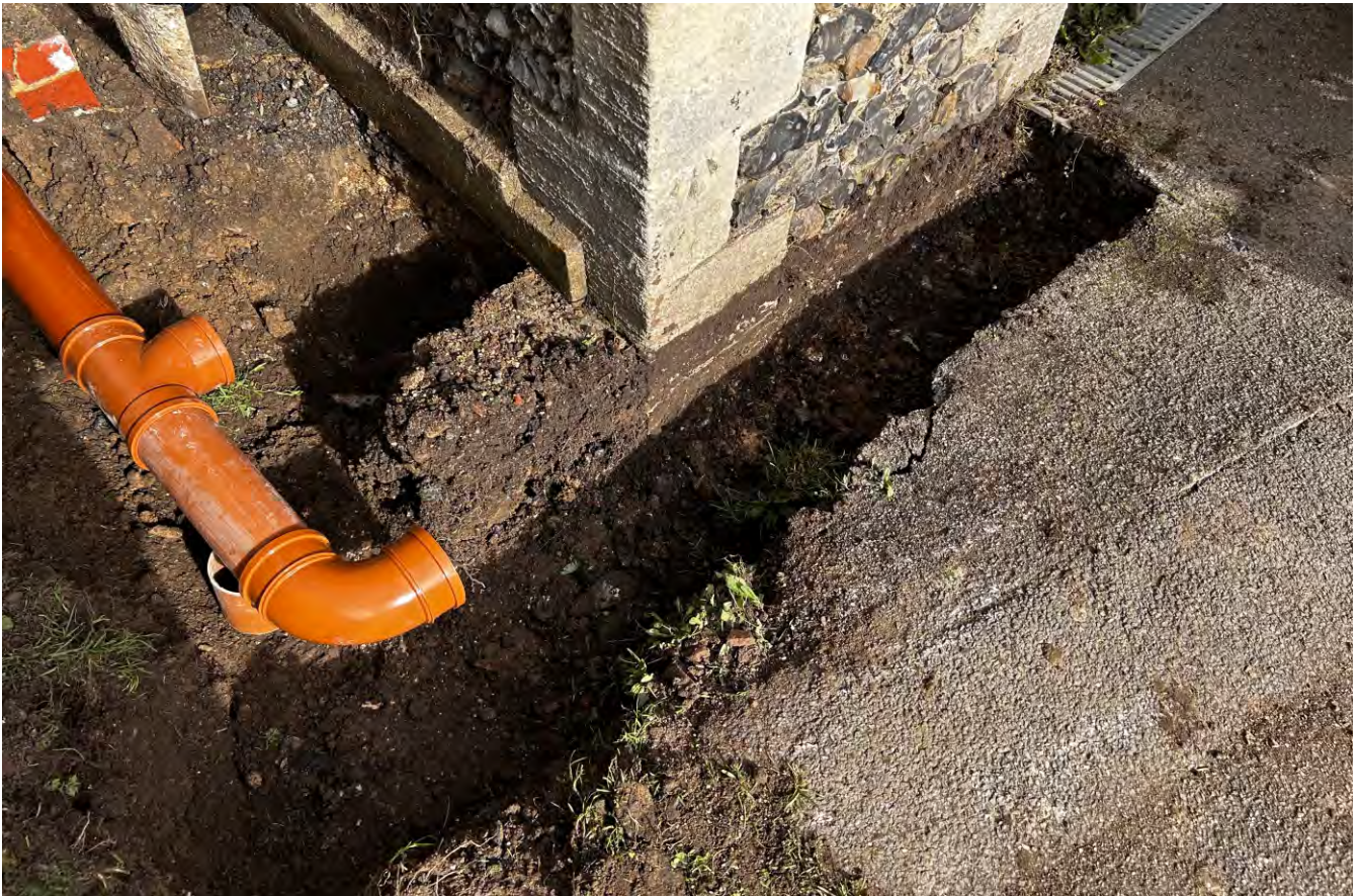
Plate 9. Detailed view looking northeast showing the southern end of trench 2 connecting with the slotted drain across the threshold of the South porch door (top right) ( note: concrete foundation addition to the porch's southern wall base ).
