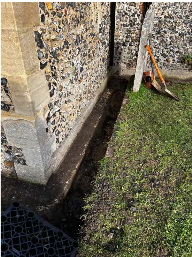
Plate 8a. Detailed view looking along the line of Trench 3 showing C.19th concrete porch foundation addition.
