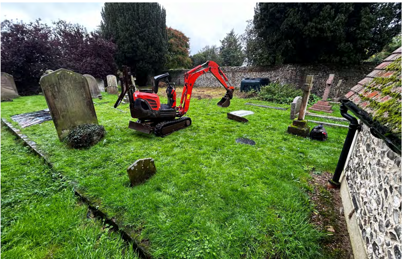
Plate 2. General view looking northeast from the north side of the church across the site of Trench 1 and Soakaway 1.
