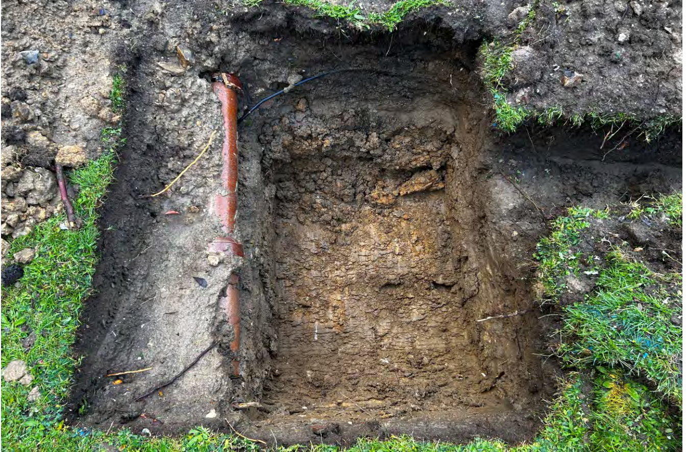
Plate 15. Detailed view looking into Soakaway 2 during its initial excavation showing ceramic drain to earlier drainage system causing the soakaway excavation position to move to the west.
