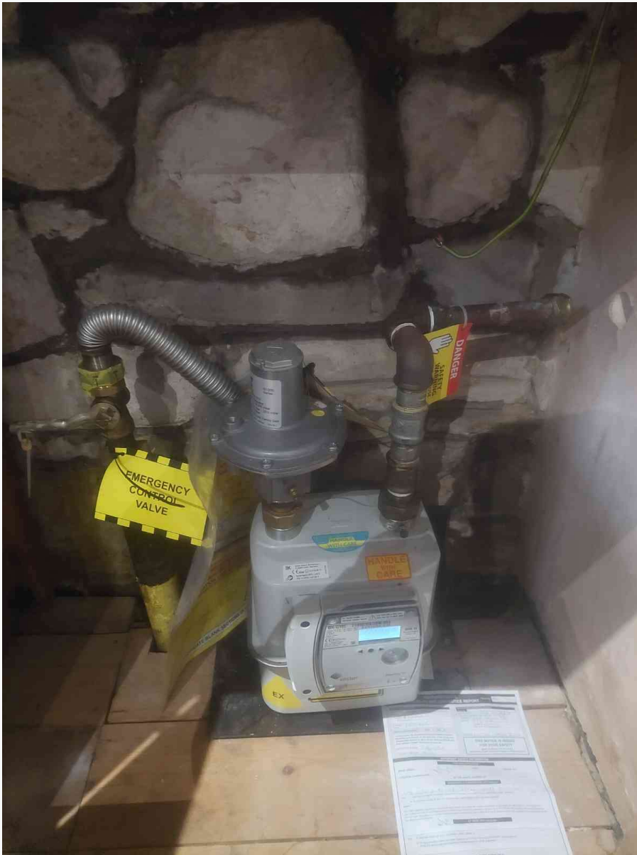
Take Photo of Existing Installation
