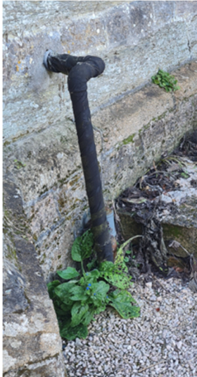
Mains Gas Installation
