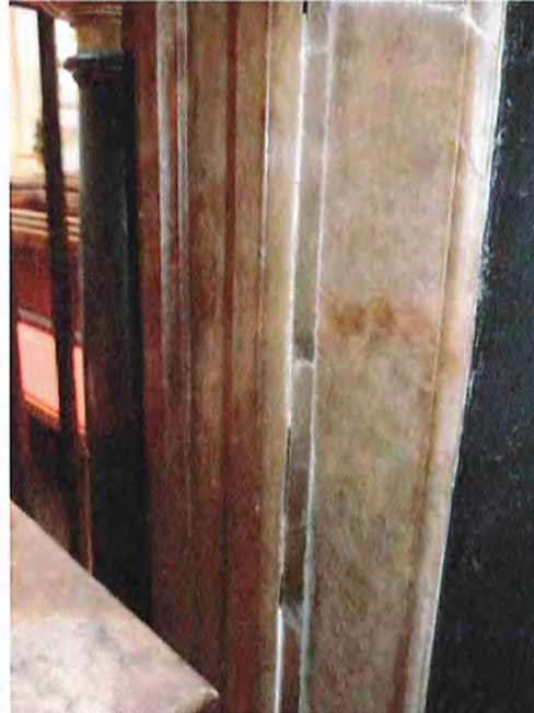
Fig 10: detail of indents on frame
