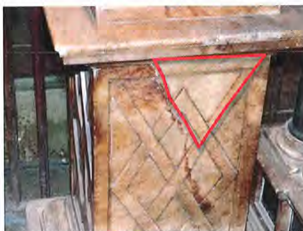
Fig 37: area of plinth showing effect of light clean with melamine sponge
