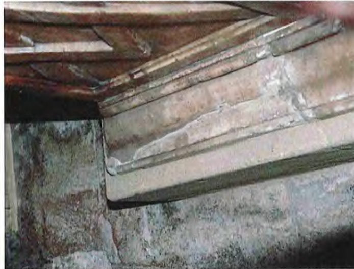
Fig 29: detail of lower moulding on SE corner showing section made up in plaster
