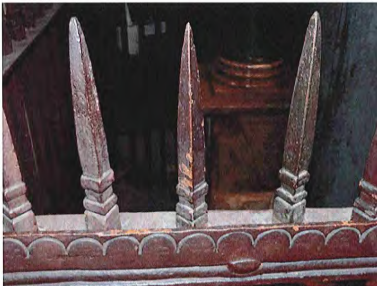
Fig 34: detail of paint loss from railings showing red oxide beneath
