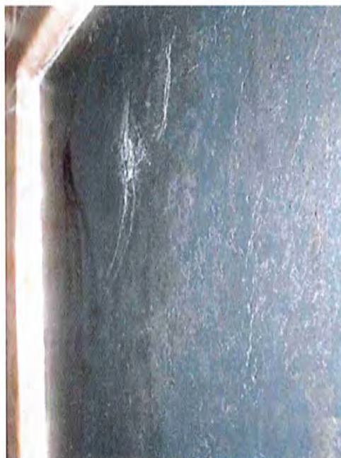
Fig 11: condensation on east end panel
