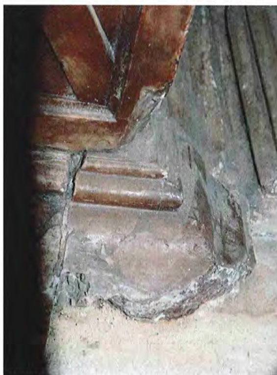
Fig 28: disrupted stone at base of plinth (NW corner)
