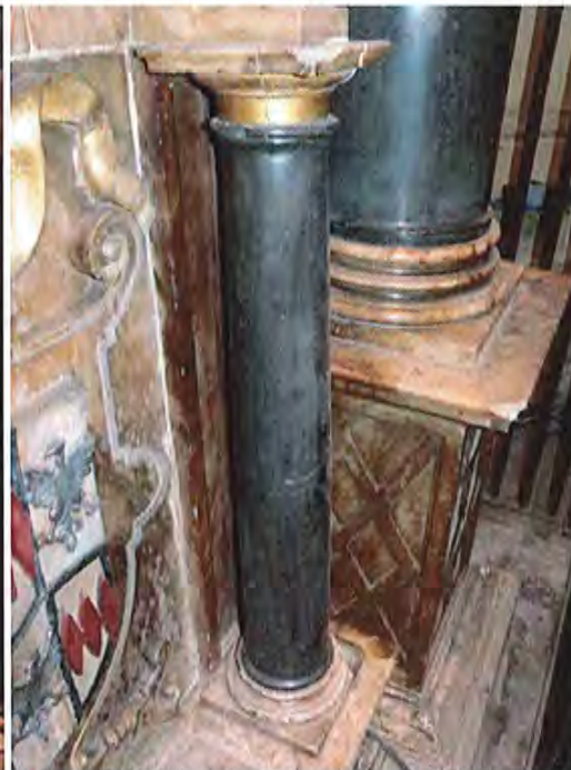
Fig 8: SE corner column showing some milkiness on the surface
