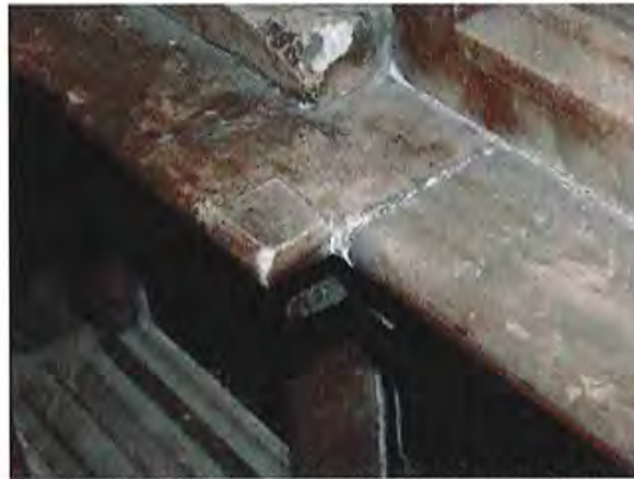
Fig 5: detail of typical indent on the top moulding of the plinth
