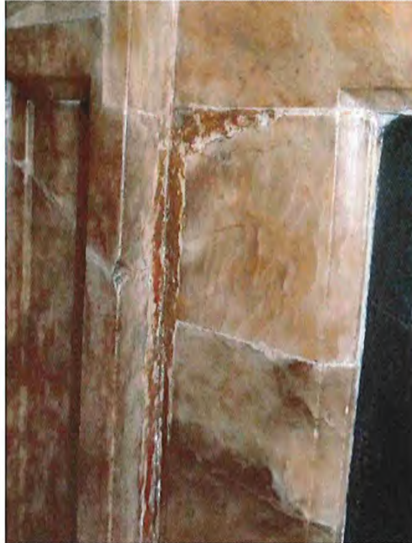
Fig 3: detail of west end panel showing pigmented wax applied to the surface of repair/pointing
