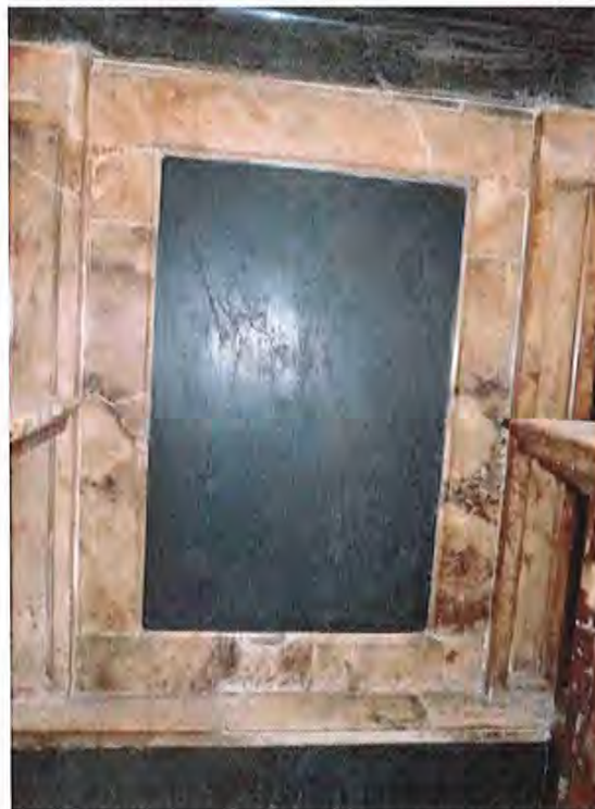
Fig 2: detail of west end panel with indents and repair visible on the frame
