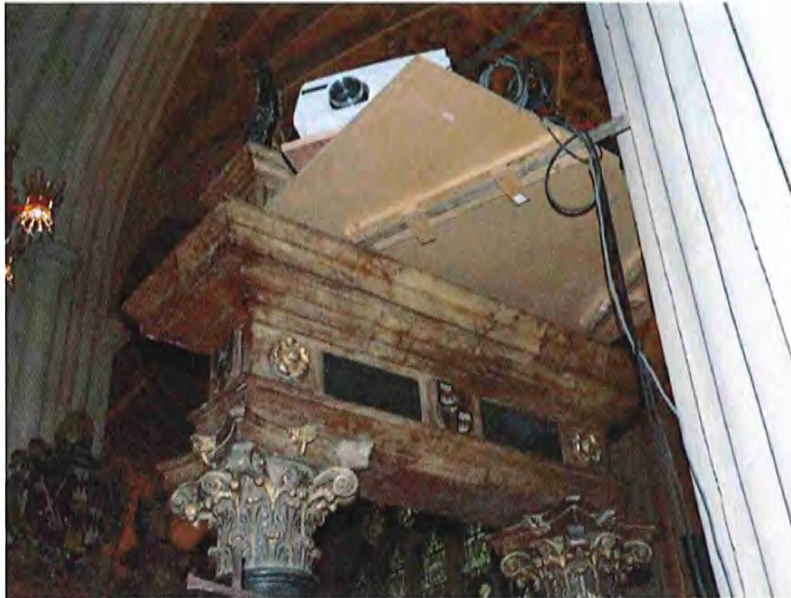
Fig 31: detail of east side of east entablature showing how it is being used as a projector stand
