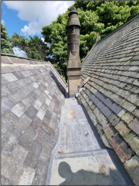
Original lead flashings around the chimney, and in the adjacent section of gutter have been kept.
