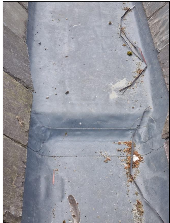
Package straps left in the gutter to be removed.
