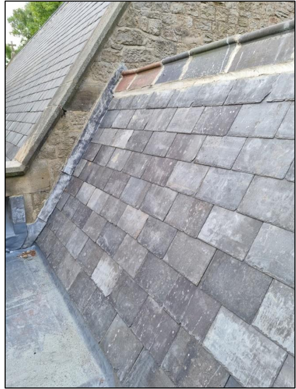
Looking east at north pitch of the vestry roof. Imported Welsh Slate has replaced the Westmoreland which was in poor condition.
