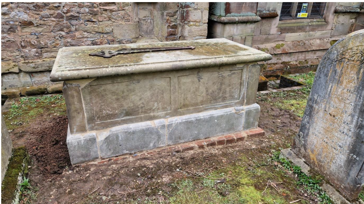
Plate 14: the stone top to the memorial was then maneuvered into position utilizing an A-frame and lifting equipment. The lid was placed onto the same bedding mix as the rest of the tomb stones.
