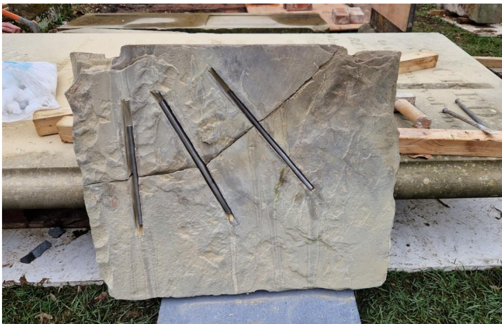
Plate 10: this is the rear of the west end panel. The stainless steel dowels are set into pre-cut grooves.
