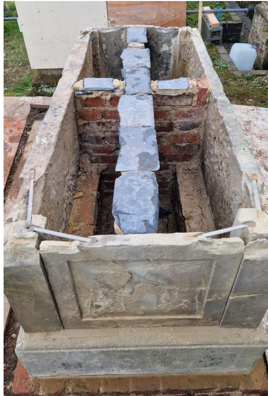
Plate 13: the panels are now bedded down and cramped together. The brick core was built up with slate packers to bring the core level with the outer panels. Although all of the good core material was used up it was necessary to include 25 new bricks. The new bricks were supplied by Bulmer Brick and Tile company, Sudbury.
