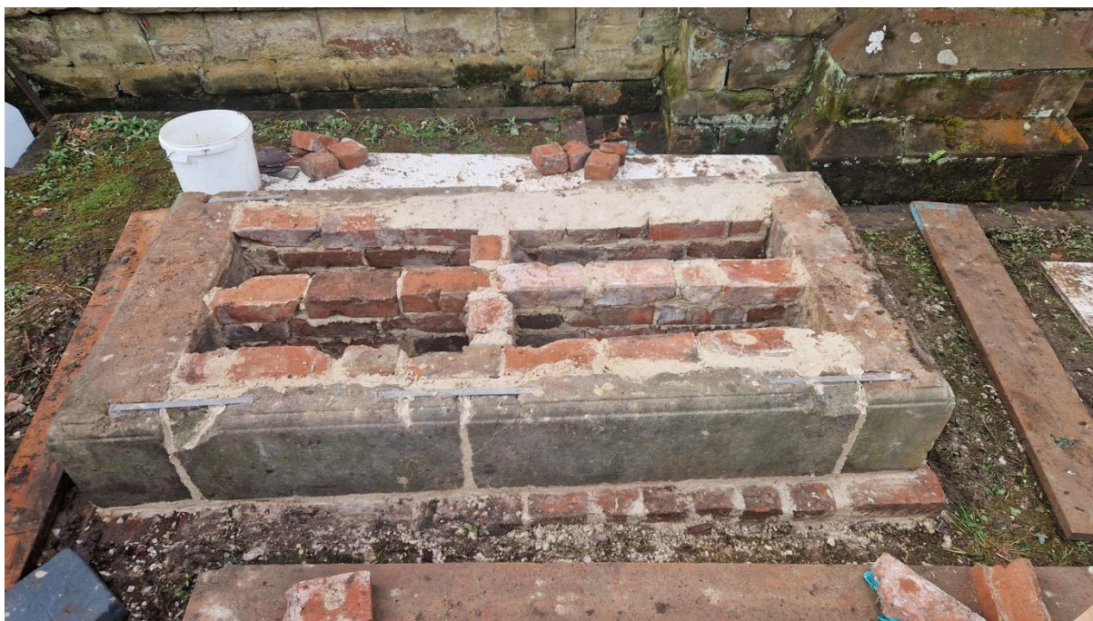
Plate 12: here we can see the plinth stones in position and cramped together. Also the brick core was built up in the same arrangement as the original.
