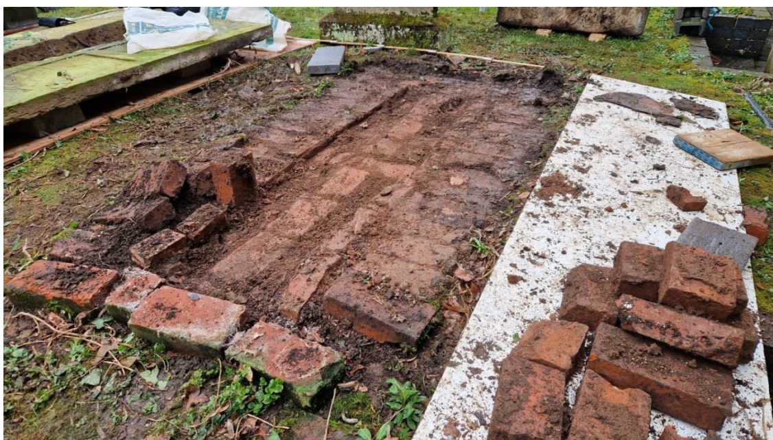
Plate 11: showing the disruption to the brick foundation.
