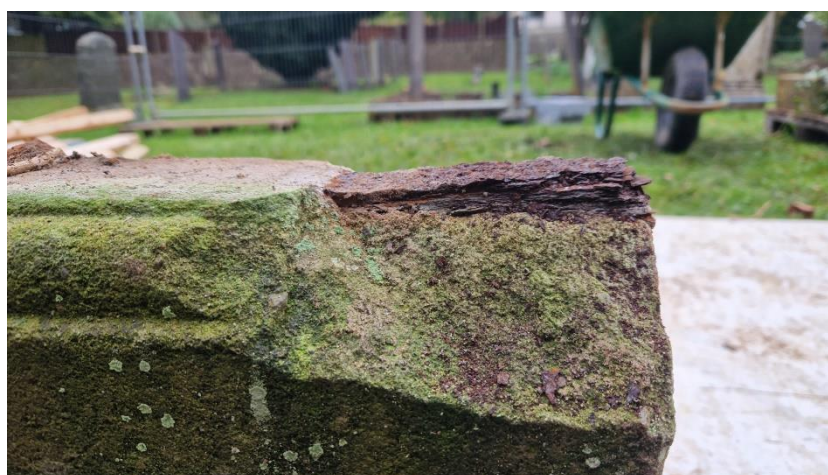
Plate 8: here we can see the level of delamination to one of the plinth stones iron cramps. This delamination has caused the surrounding stone to fracture and break away.
