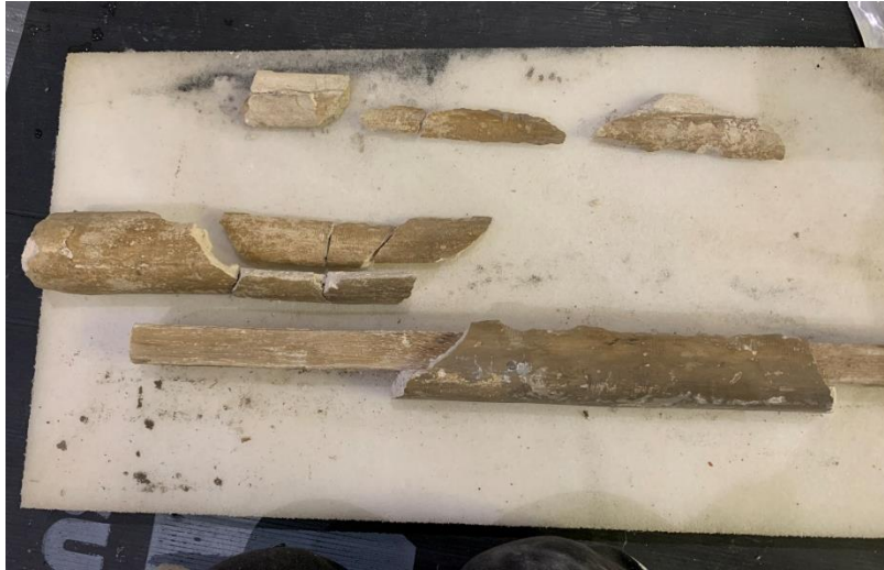
Plate 8: The loose bullnose moulding and plaster sections from the west face.
