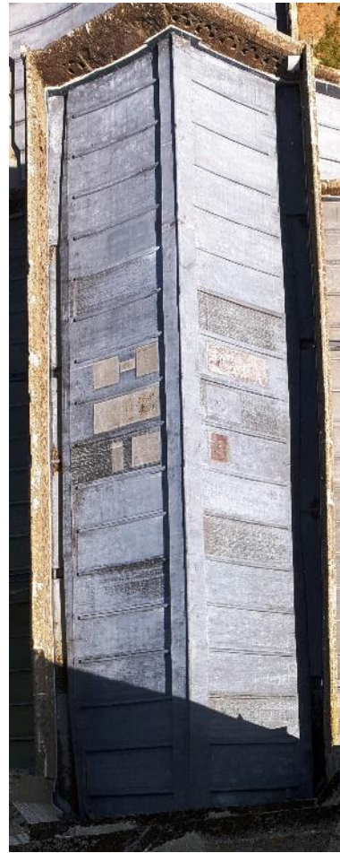
Figure 21A: Nave Roof showing graffiti
