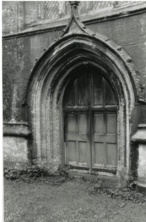
Figure 2: Double door access to west tower – these are in poor condition and cannot currently be opened
