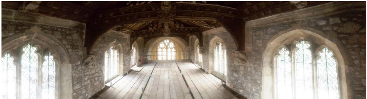
Figure 23: The Nave ceiling with the iron tie bars removed and windows restored.
