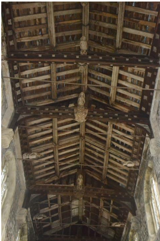
Figure 10: Nave roof showing roof beams and ornamentation. The 5 th Truss and iron tie bars that were removed during 2018 nave roof repairs are also visible.
