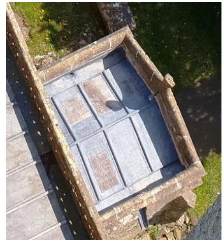
Figure 21B: Porch Roof showing graffiti
