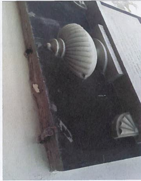
Rusting and displaced restraint cramps at top
