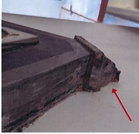
Supporting corbel has hairline crack, not visible here.
