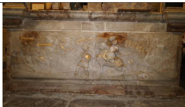
Fig. 23: battle scene panel with visible open joints, cracks, deterioration of stone in lowest part, discolorations
