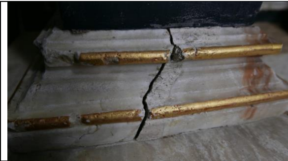
Fig. 31: open crack previously repaired with plaster
