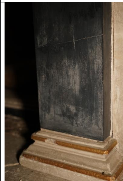
Fig. 35: discoloration of the black marble column shaft
