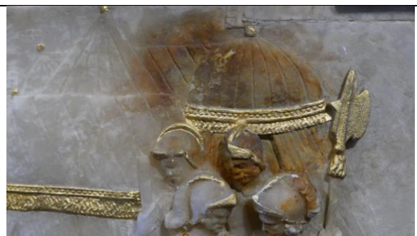
Fig. 24: ferrous stains in top right corner of the panel
