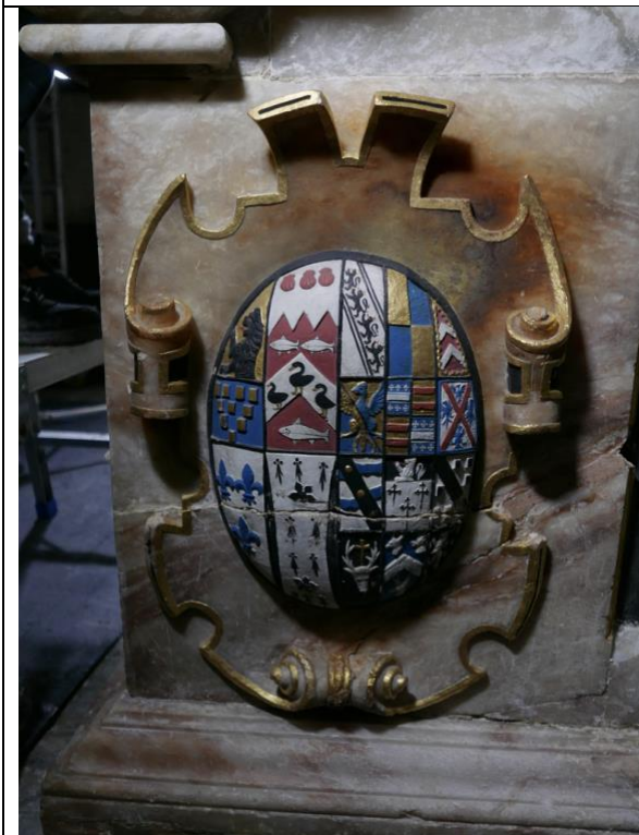
Fig. 45: coat of arms with horizontal fracture across the shield; noticeable ferrous staining of the alabaster
