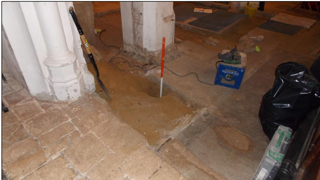
Figure 21. Exposed section of concrete in North Aisle, 1m scale
