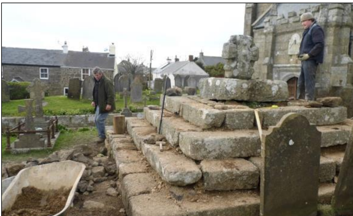
Fig 31 Conservation work in progress: the use of rab (local orangey-brown granitic subsoil) to level the stones can be seen in this picture (in the stonework joints and in the wheelbarrow) (AGL).
