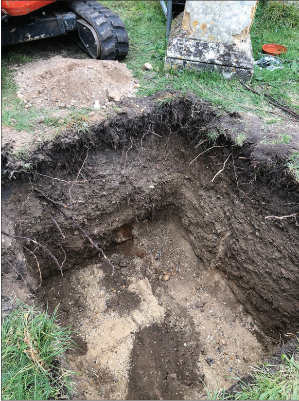
Plate 7: The soakaway at its final depth of 1.6m, showing cut of grave 1 (foreground) and grave 2 (background), looking south-east
