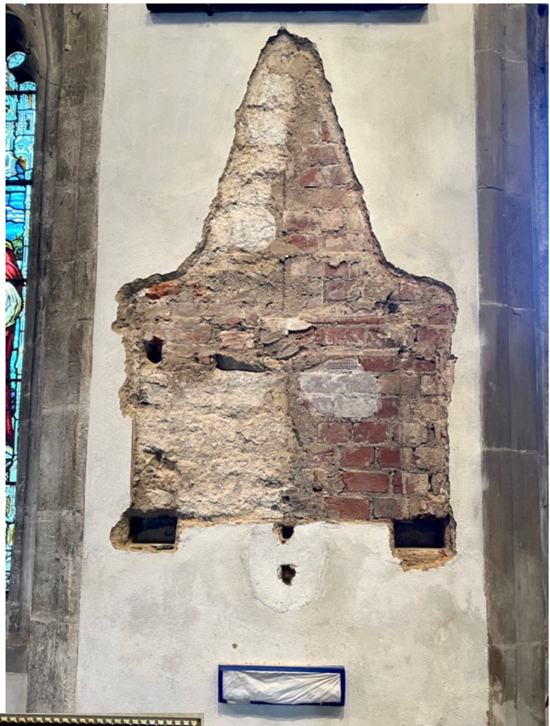
Figure 27 ~ North elevation after monument to John Gordon dismantled. Areas of historic painting and greek inscription are faced up with tissue as protective isolating prior to replastering.
