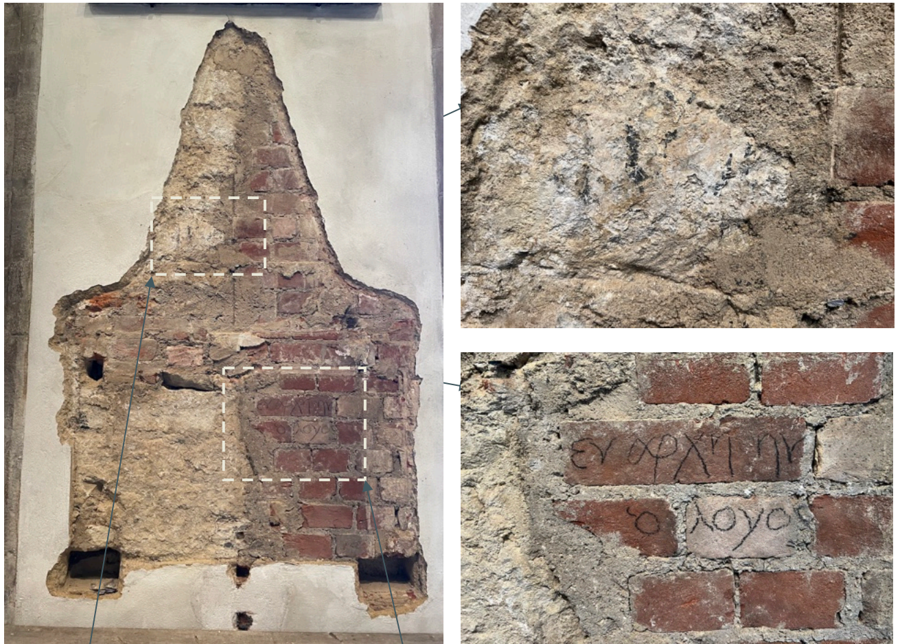
Figure 26 ~ North elevation after removal of Gordon Monument, illustrating location of historic painted inscription, A, and more recent, 2000, inscription, B.
