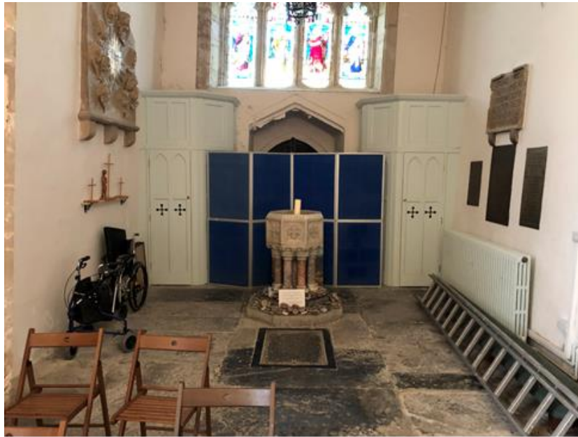
Image 1 – View of the base of the tower showing the existing cupboard enclosures either side of the unused west door.
