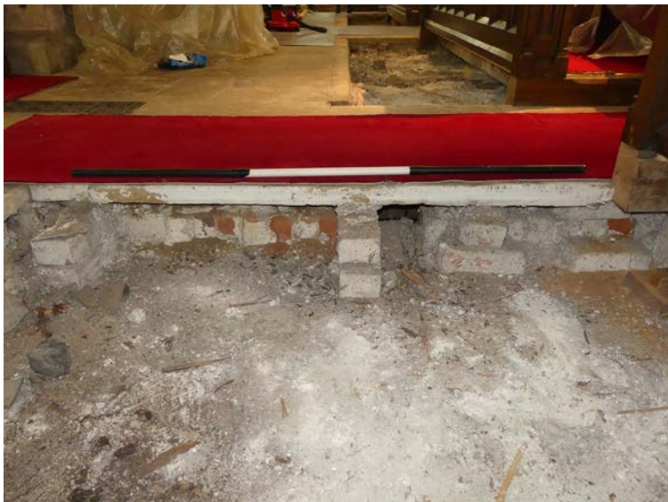
Plate 13: Bricks below the flag floor on the south side of Area 4, viewed from the north
