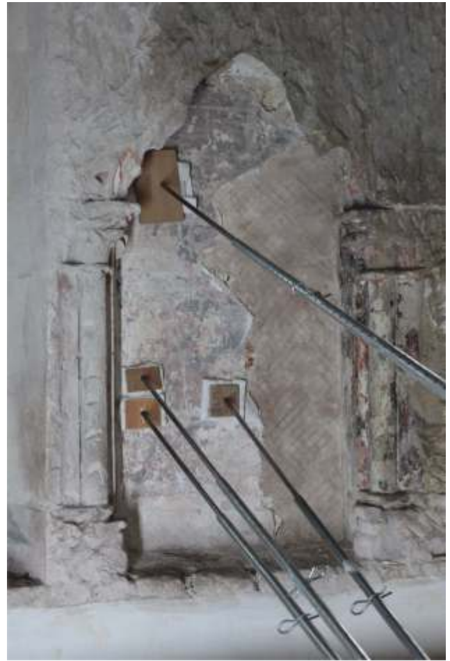
6 - Above - Base coat plaster on RHS as well as further securing detached plaster.
