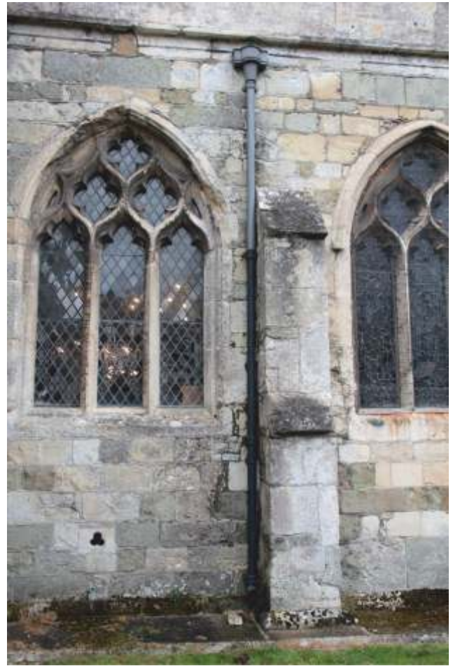
2 - Above - Exterior fabric 2022 with repaired downpipe.
