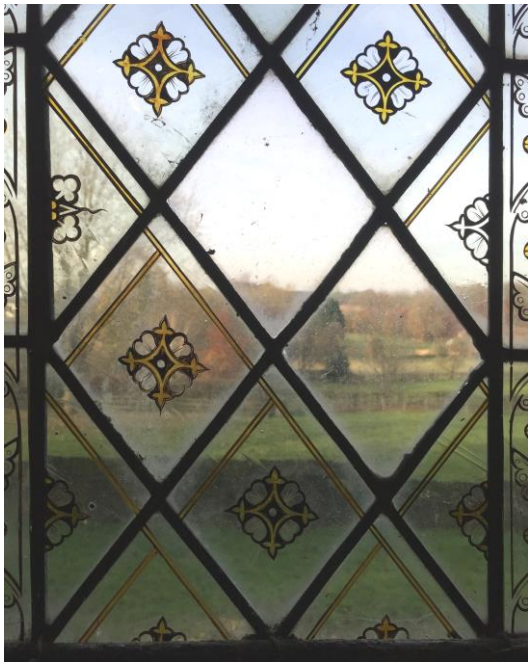
Detail: window nV light b before restoration showing previous unpainted repairs
