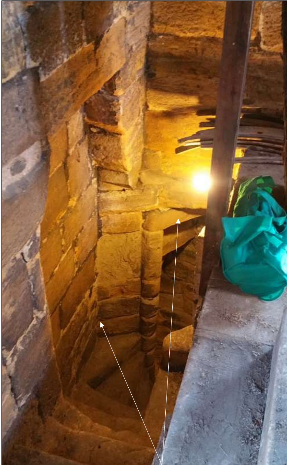
Plate 9. Top of spiral stairs showing continuation of now blocked of spiral (D Beaumont)
