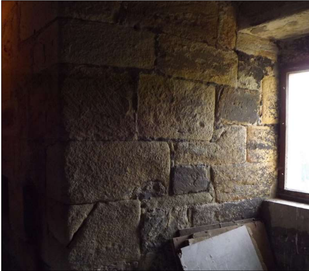
Plate 8. Irregular stone work in window reveal
