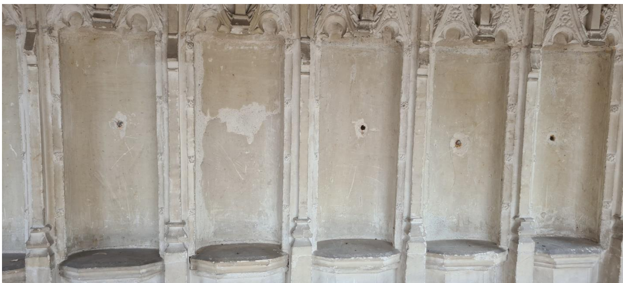
Plate 15: Historic iron fixings before removal
