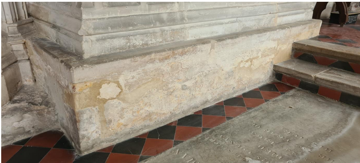
Plate 30: Base of tomb chest (south side) consolidated with lime putty repair mortar mix
