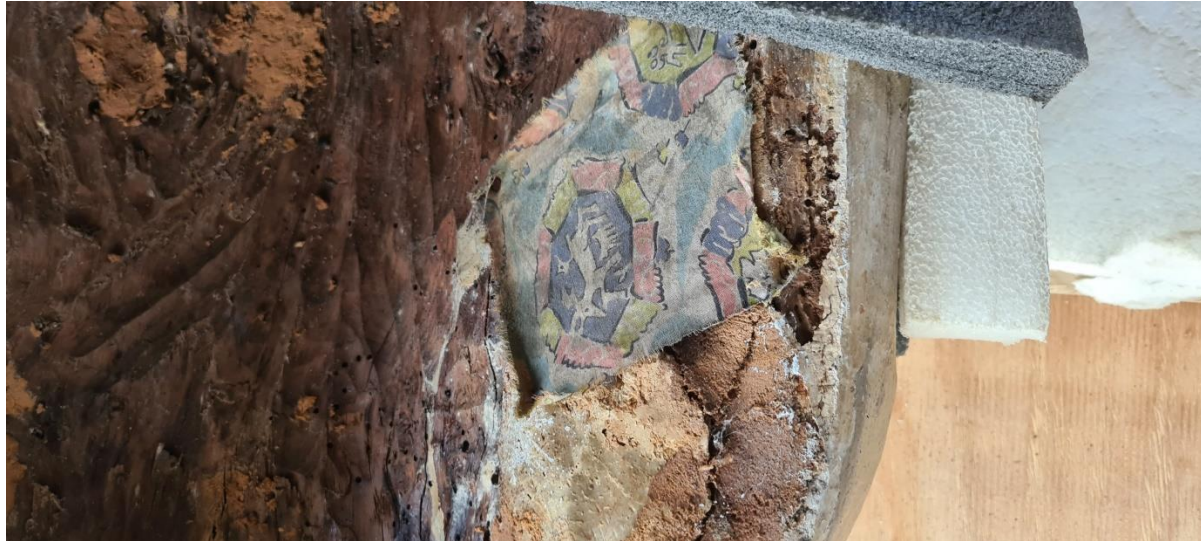
Plate 34: Material used to repair insect damage underneath Katherine de la Pole effigy
