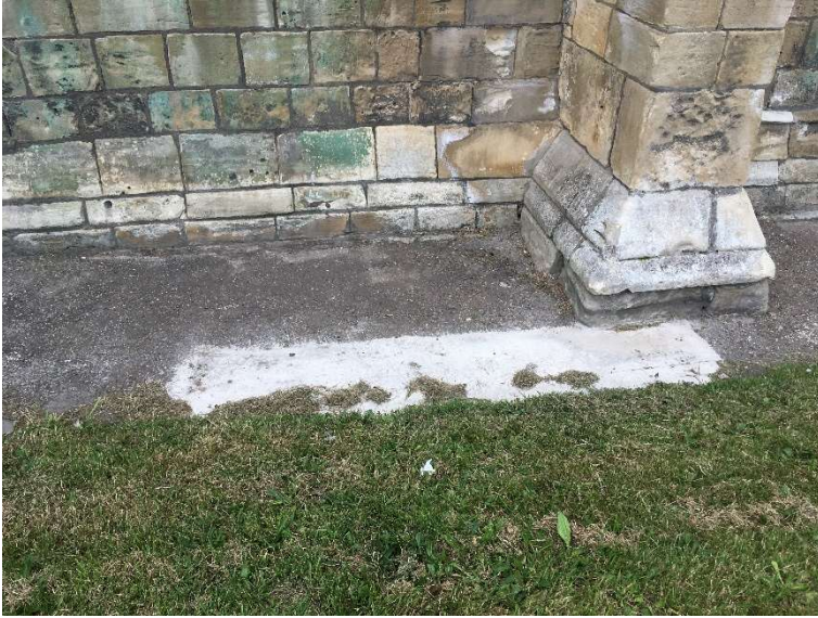
Broken concrete repair, there was no pipe below.
