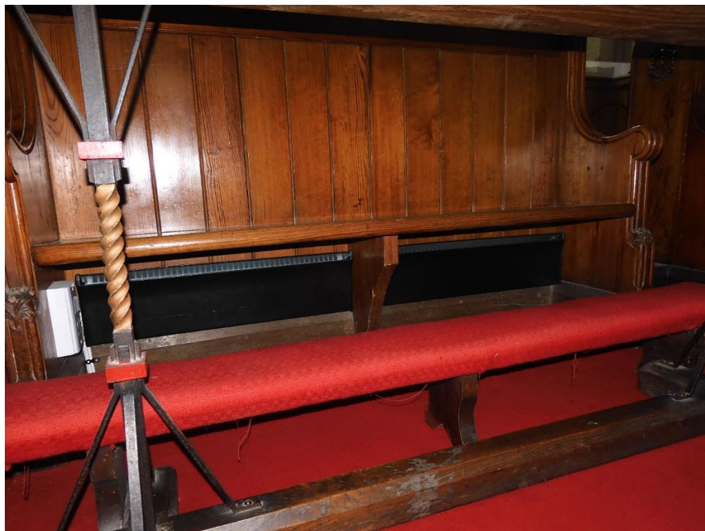
Black 650W Norel under pew heaters fitted to solid pew backs.
