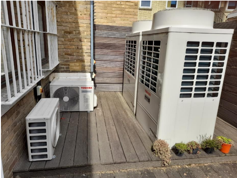
Examples of external units for AASHP comprising of three smaller 3kW units and two larger 10kW units.
