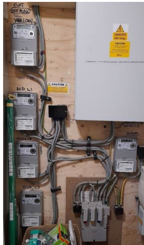
Hall, office and flat meters
