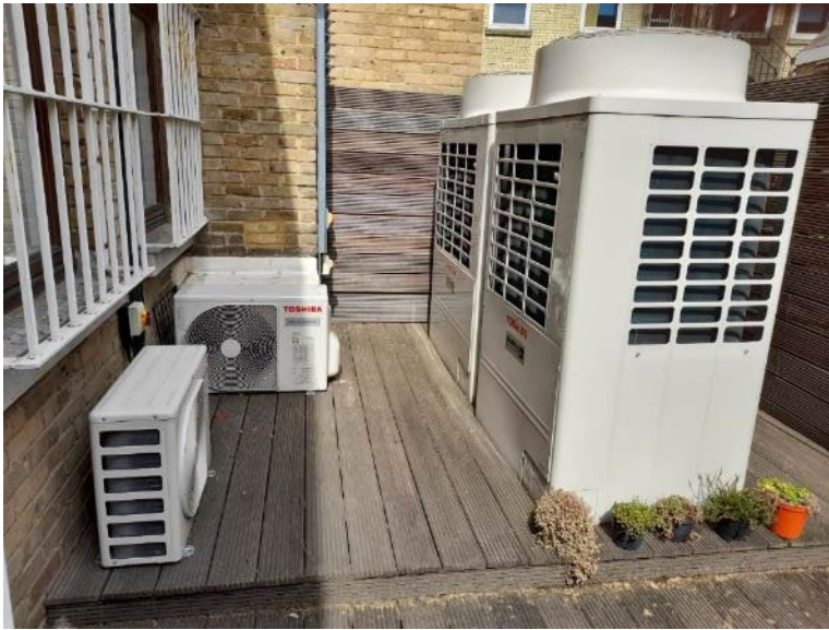
Examples of external units for AASHP comprising of three smaller 3kW units (10kW output each) and two larger 10kW units (37.5kW output each).
