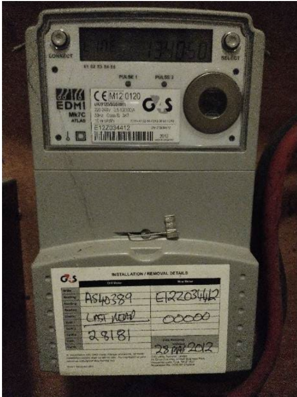
Church electricity meter
