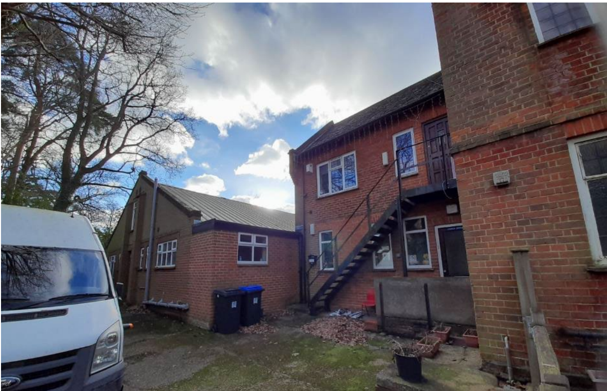
East end of site showing the end of the hall (elevation containing meeting room and toilets), link block to ground floor office, external stairway to first floor flat, end of church to right.
