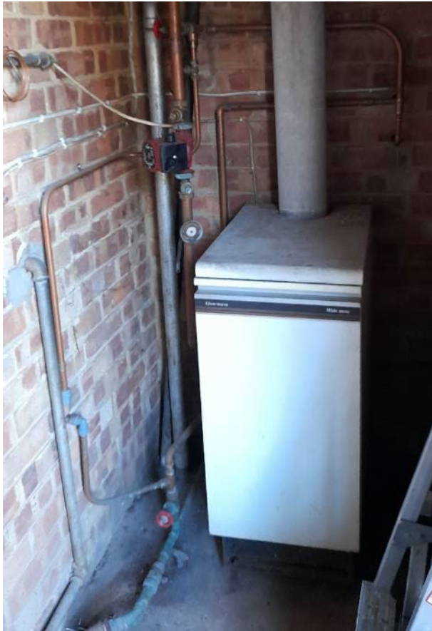
Hall Glo Worm boiler
