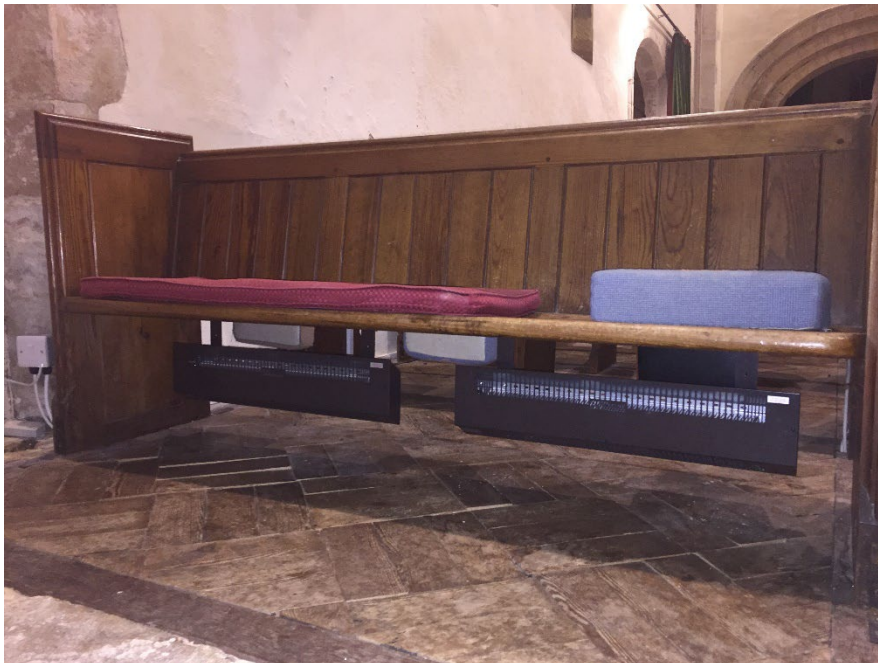
Brown BN Thermic 650W under pew heaters fixed to underside of pew seats for pews which have no solid backs.
