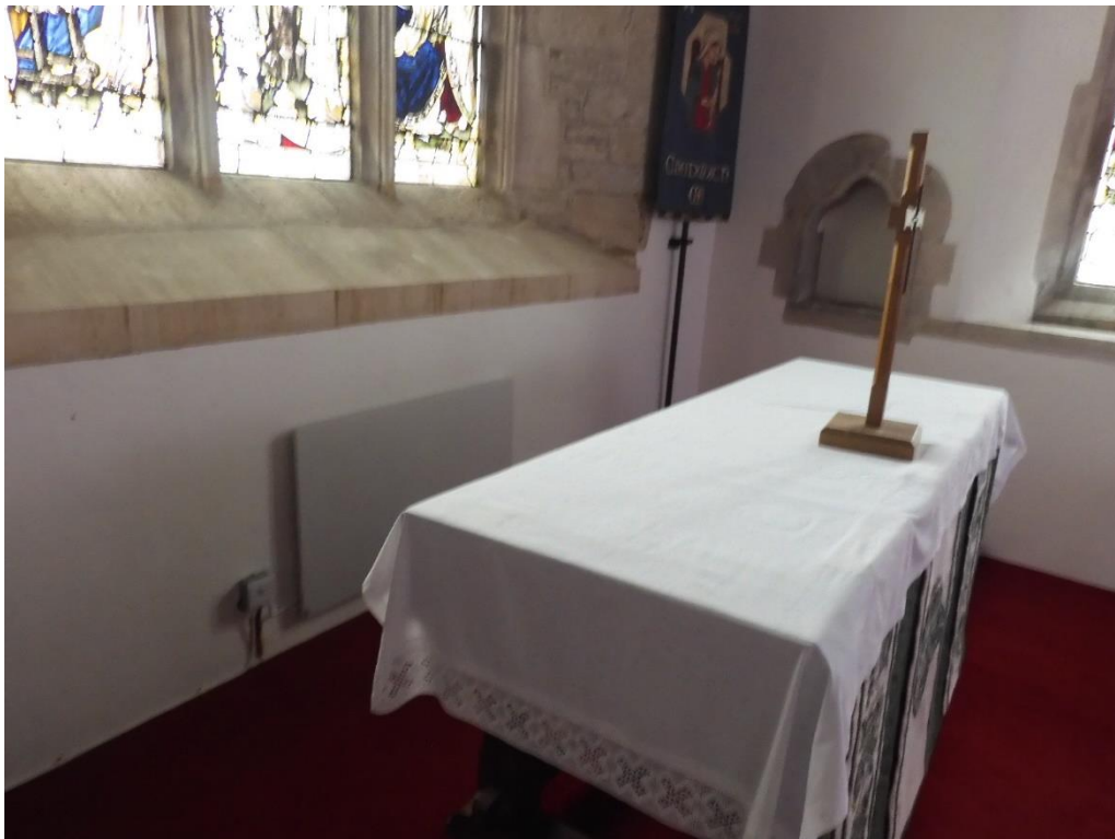
Electric panel heater installed behind an altar
