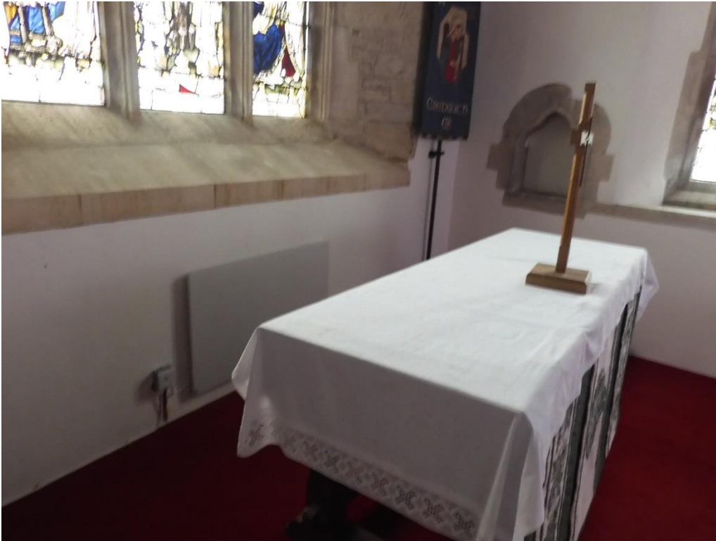
Electric panel heater installed behind an altar
