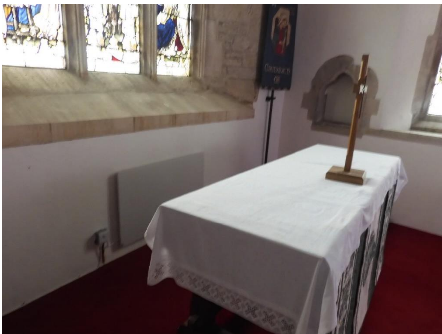
Electric panel heater installed behind an altar
