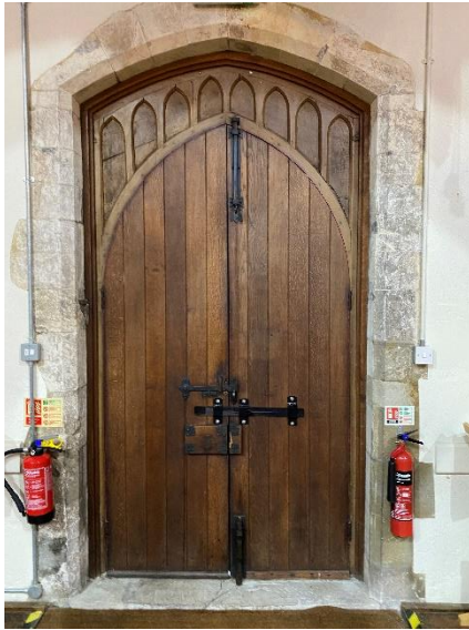
West facing door which should be considered for installation of overdoor heater.
