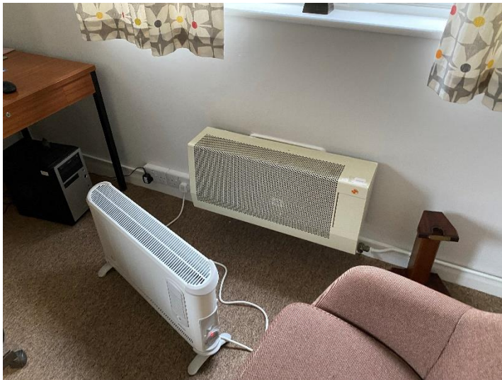
Existing radiator in vestry which is one area considered for replacement.
