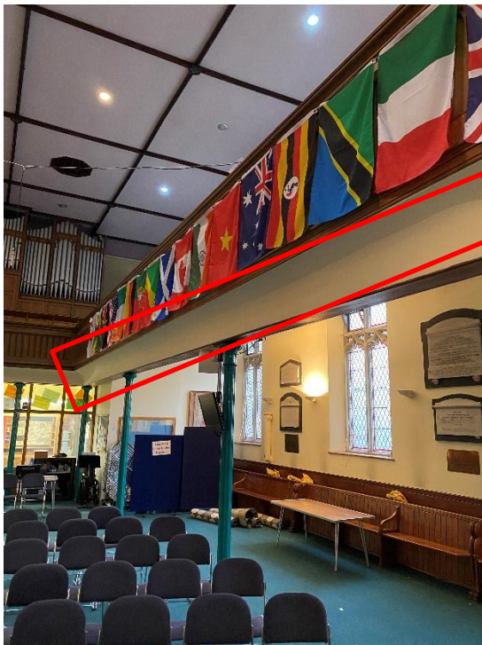
One area for consideration of installing overhead IR heaters
