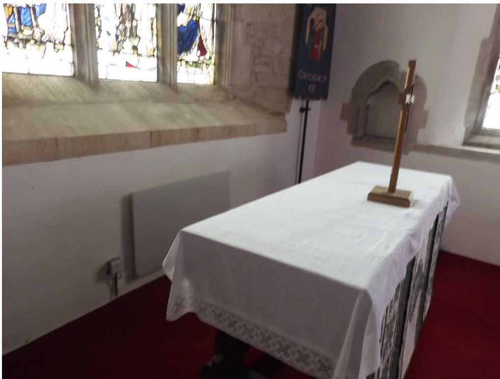
Electric panel heater installed behind an altar
