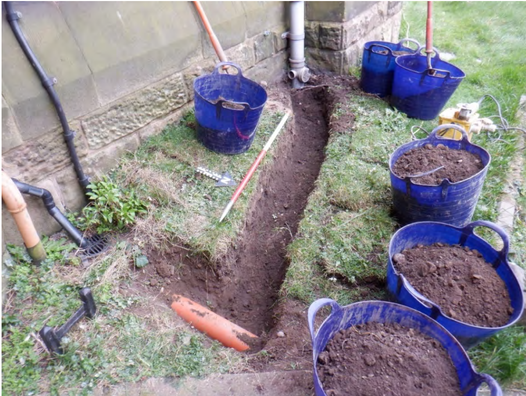
Figure 3: Photograph showing the excavated area. Looking south-west, scale 1x1m in 0.5m graduations.
