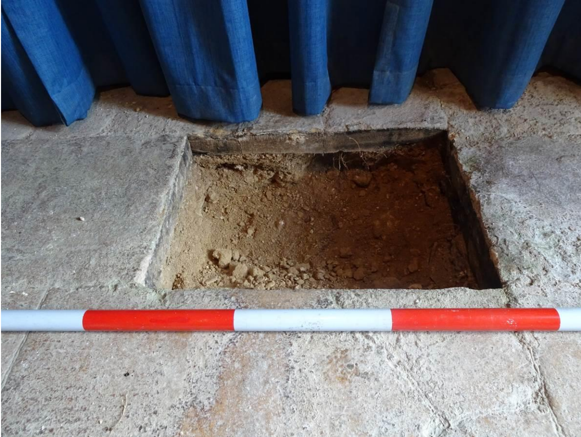
Plate 5. Trench 1. Excavated subbase material within tower floor to desired depth, looking north
