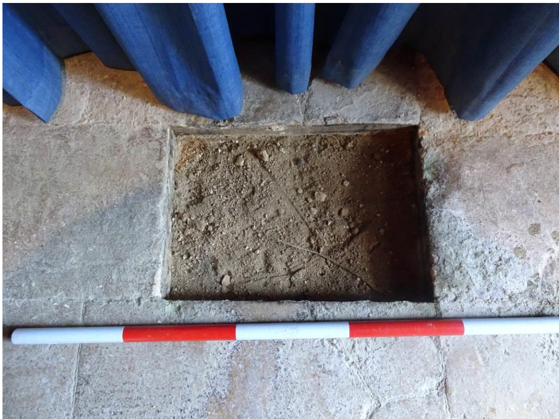
Plate 4. Trench 1. Exposed subbase material within the tower floor, following removal of flagstone
