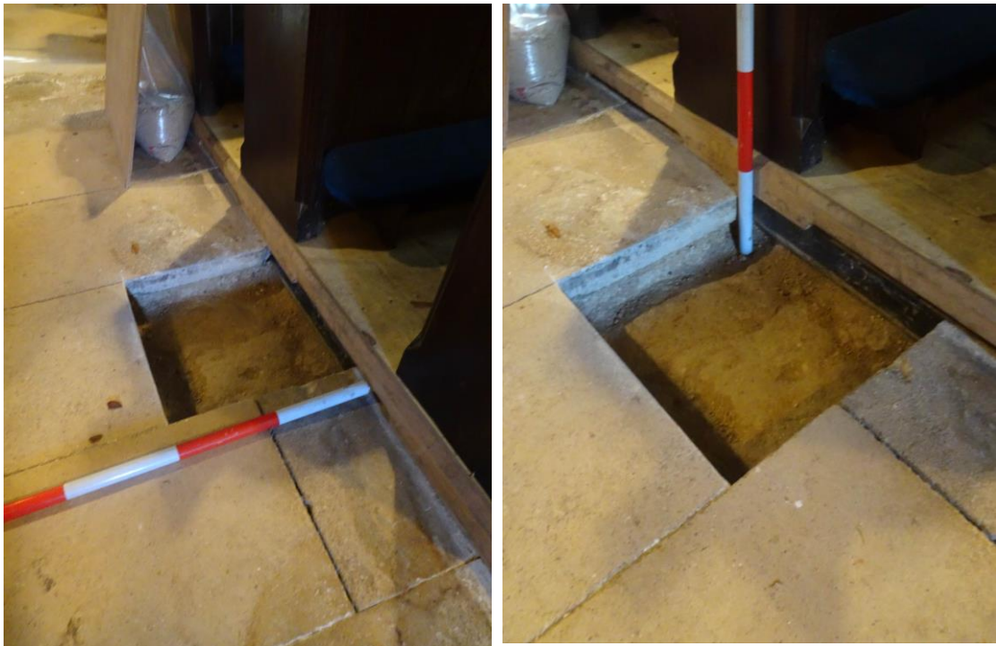
Plate 8. Trench 3 (central Nave). Small trench revealing the subbase material Plate 9. Trench 3 (central Nave). Excavated subbase material to the desired depth
