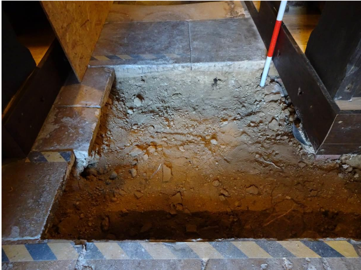
Plate 7. Trench 2. (Western Nave area) Excavated subbase to the desired depth, looking east
