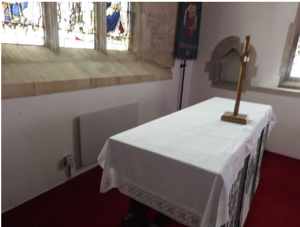
Electric panel heater installed behind an altar
